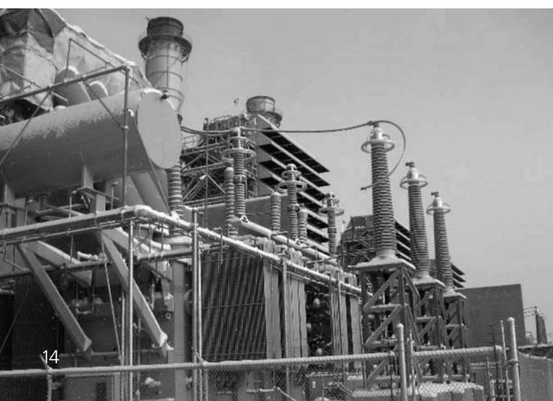
Top: Installation of lattice steel structures for interconnection of the Port Alma Wind Project, near Leamington, to the transmission system.
