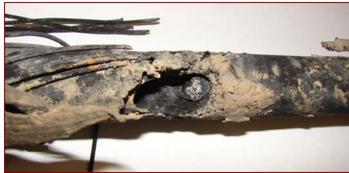
Figure 1, Aluminium core melted from failure
