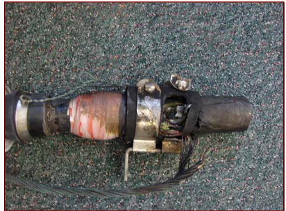
Figure 2, Cable fault on the 19M26 (2008)
