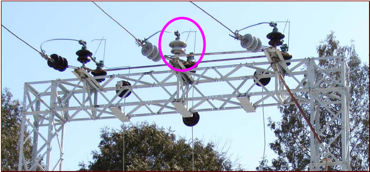
Figure 1, Gang operated switch 35T1-L
