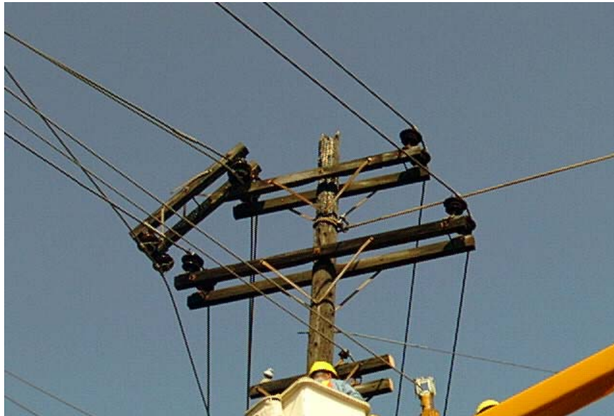
Figure 19, Pole Fire Damage
