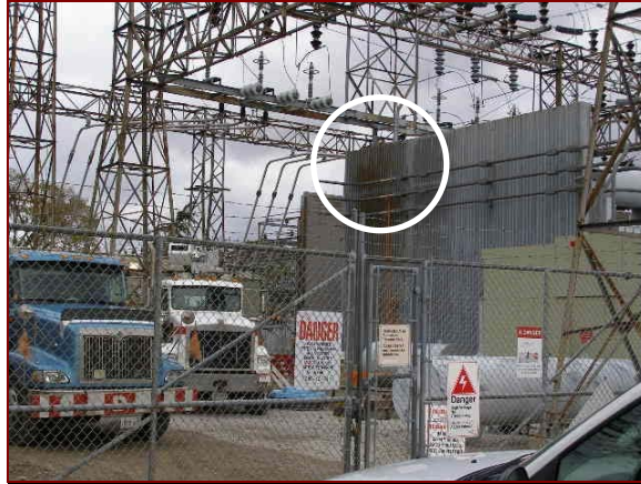
Fig 4 – Separation wall affected by the failure of T4
