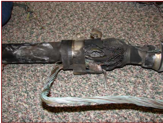
Figure 1, Cable fault on the 19M25 (2007)
