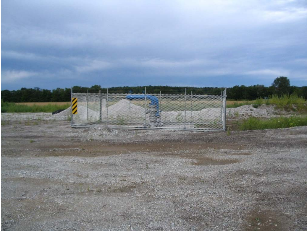
Photo 1 – TW#13H; looking west
