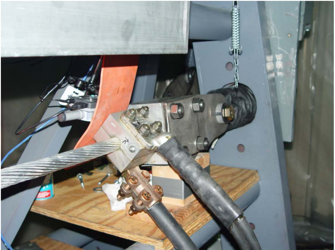
Photograph 2, current termination (foreground), and resin fitting (background)
