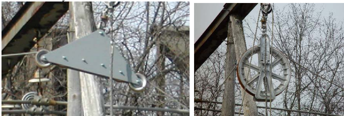
Figure 4. (a) roller array (b) single 36-inch sheave
