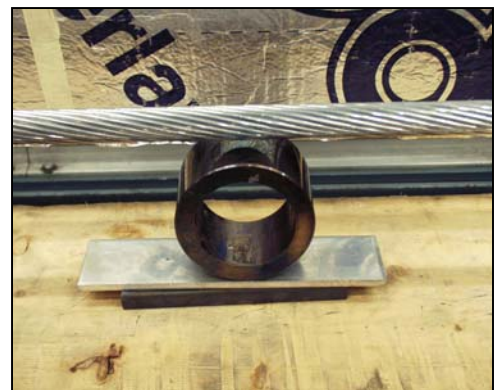
Photograph 3 Mid-span Support to Remove Sag
