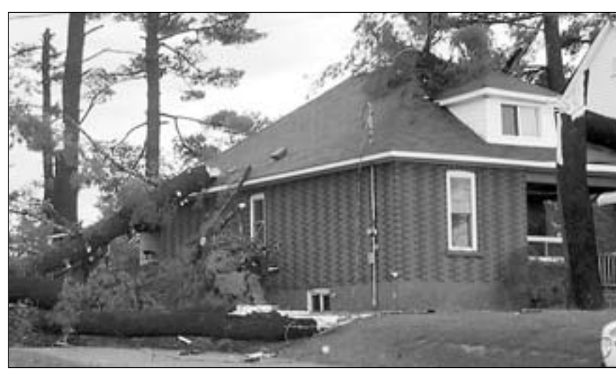
Fallen trees lean on a house at 481 McConnell Rd. in Mattawa after Monday's violent storm.
