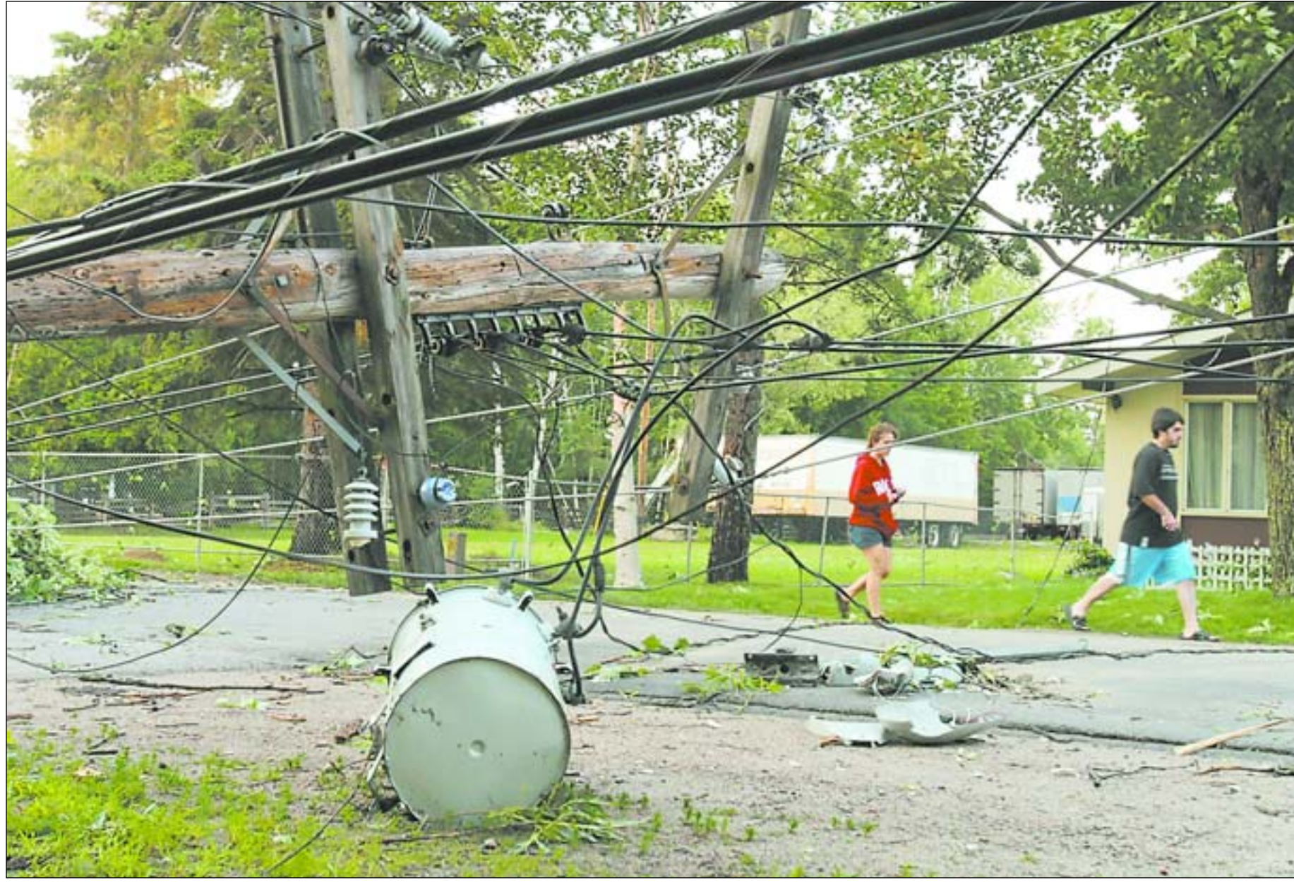
Pedestrians skirt fallen wires on Premier Road following Monday's storm that left most of the city without power. The storm hit at about 5:30 p.m., downing trees and causing severe damage. PAUL CHIVERS, THE NUGGET
