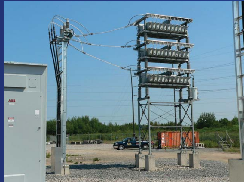
Capacitor Bank No. 5 Third Line T.S.
