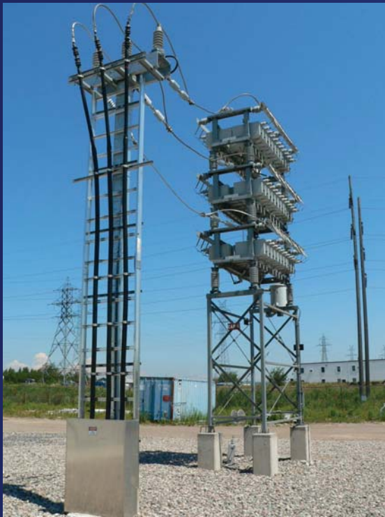
Capacitor Bank No. 4 Third Line T.S.
