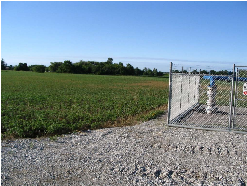
Photo 2 – TW#13H; looking southeast
