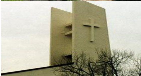
Photo above: Sequoyah Community Church, with four cell-phone antenna panels
