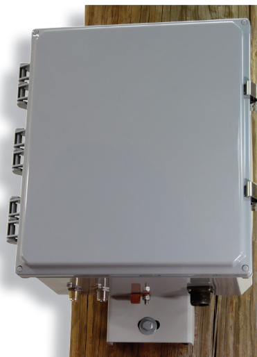
SpeedGate Utility-Pole-Mounted Radio Interface System.
