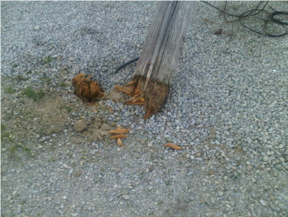
Picture 3: Pole failure due to rot at ground level.
