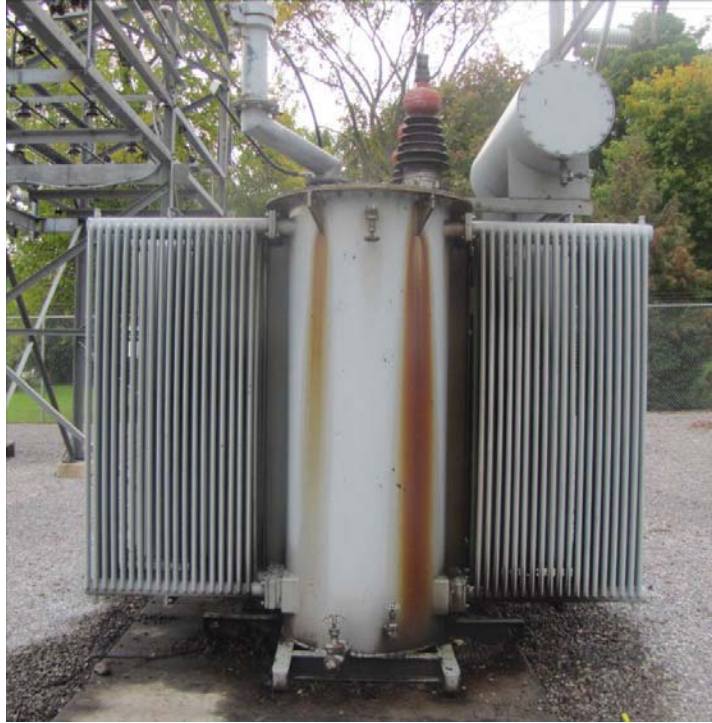
1 2 Figure 15 – Oil Leakage on a Distribution Transformer 3
