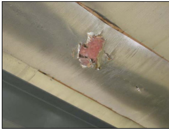
Water damage to building's roof
