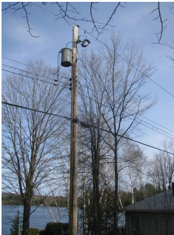
Figure 39: Typical Single Phase Pole-Top Transformer
