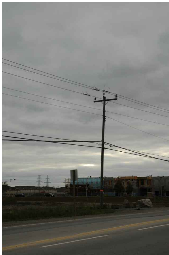
Figure 21: HONI pole with 27.6kV on the south side of Rymal Road East.
