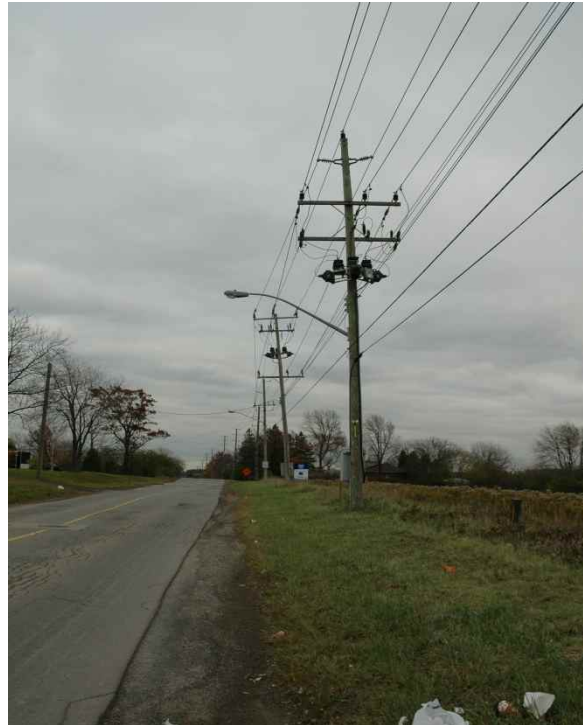
Figure 6: Demarcation point. Primary metering
