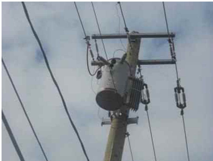
Figure 19: 4.8kV to 16kV “Rabbit” located east of Fletcher Road on the south side of Rymal Road East.
