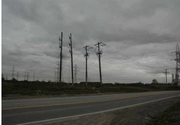
Figure 1: Express Feeders M3 and M4 tracking east out of Nebo TS and two circuits of 27.6/16kV tracking south
