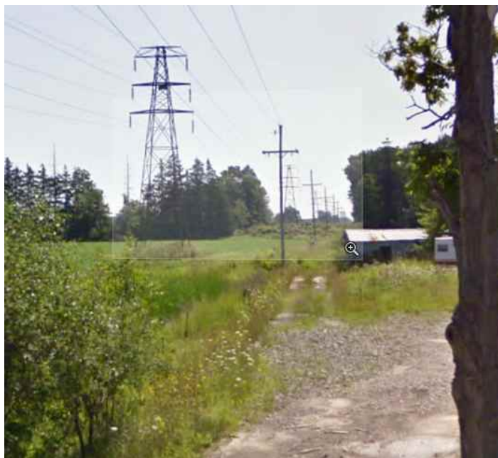
Figure 13: Rural distribution following transmission line right of way
