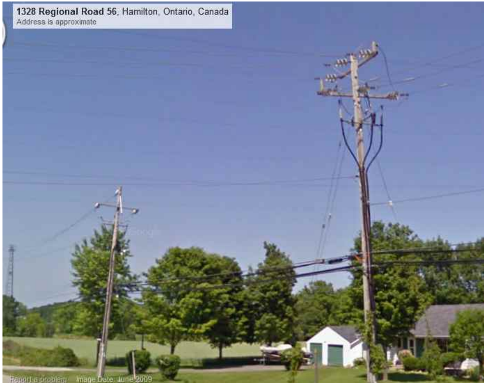
Figure 15: 8.32/4.8kV feeder reaches Highway No. 56
