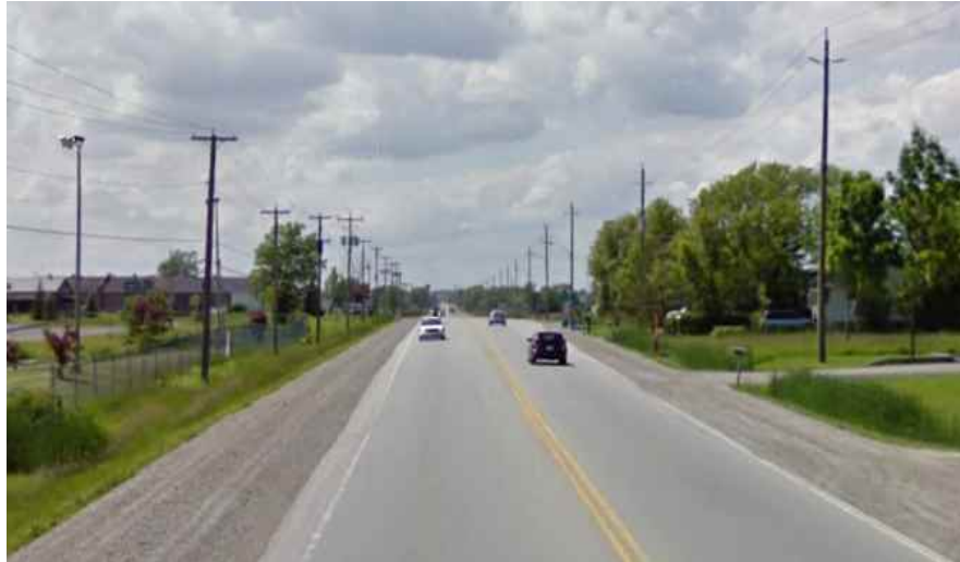
Figure 18: HONI's 8.32kV line on the south side (left) of Rymal Road paralleling Horizon Utilities' 27.6/16kV line along the north side (right).
