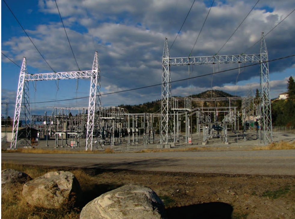
Photo 6 – RG Anderson 75/76 Line Gantry's
