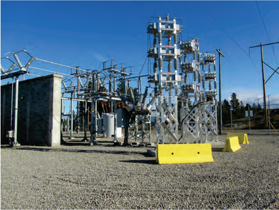
Photo 1 - DG Bell Capacitor Banks
