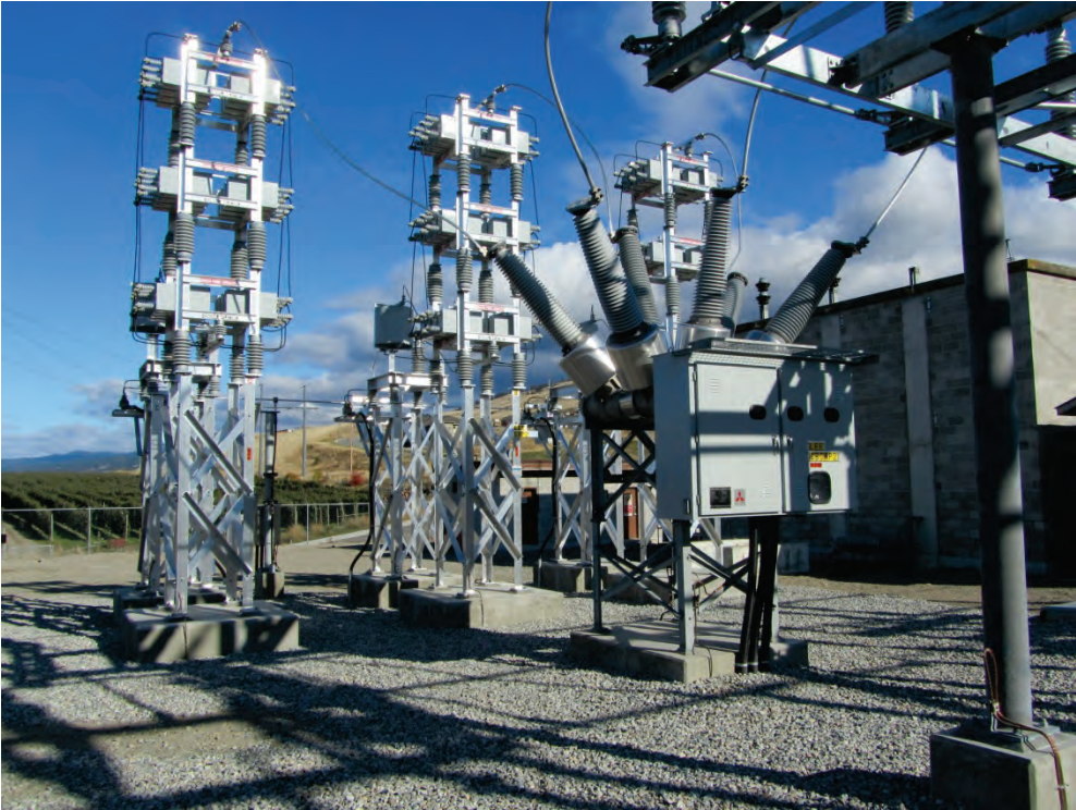
Photo 2 - FA Lee Capacitor Banks
