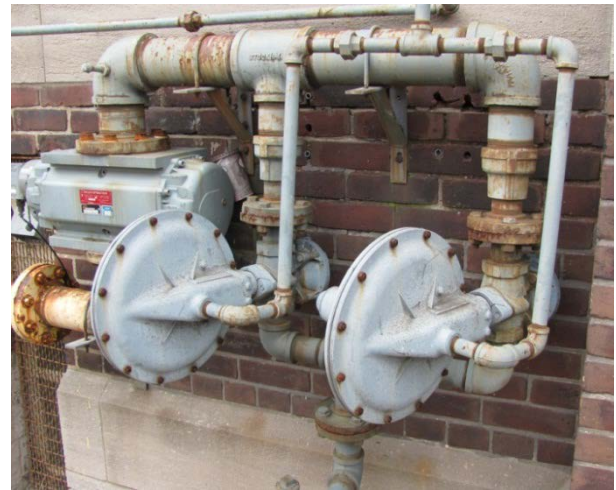
Figure 2: Rotary Meter Set with Multiple Regulators
