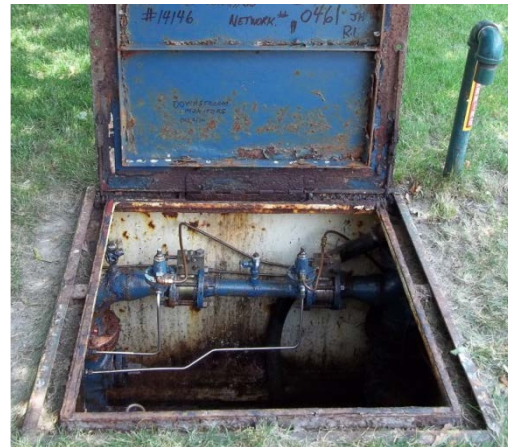
Figure 2 Condition of typical below ground district station for complete replacement.
