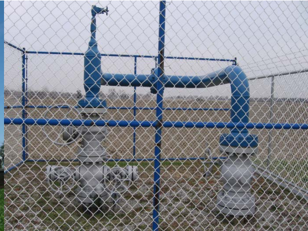
Completed Wellhead with Flow Loop and Pipeline Valve
