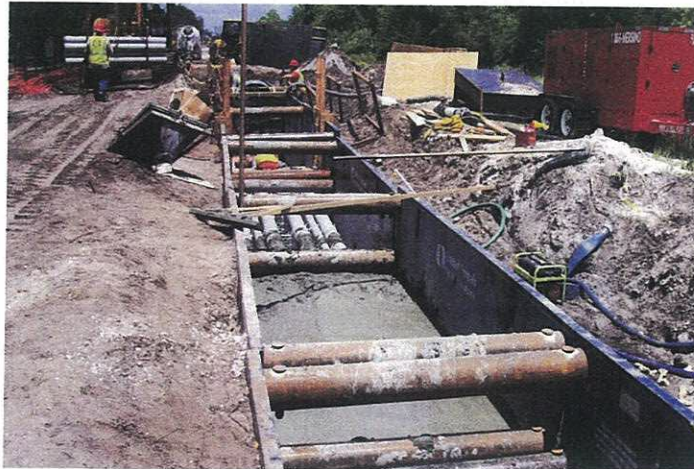
Transmission lines are installed in concrete-encased duct banks.
