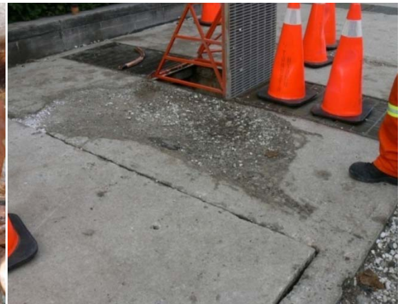
Figure 26: Cracked Vault Roof
