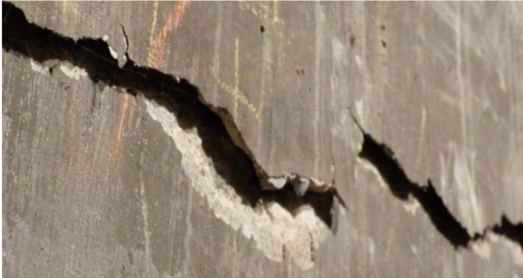
1 Figure 27: Cracked Vault Wall
