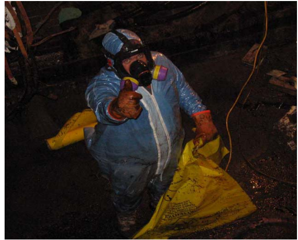
Figure 35: Asbestos clean after the fire.
