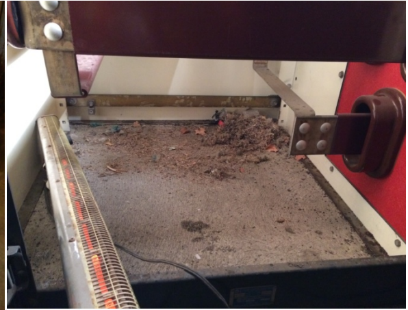
Figure 73: Pests inside Outdoor Switchgear
