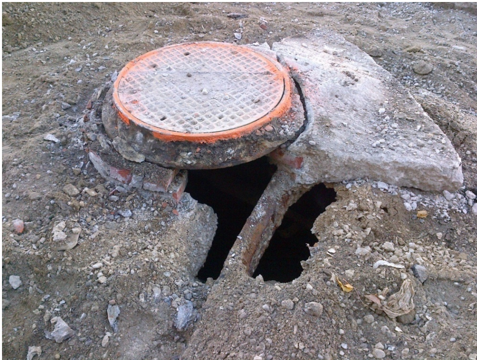
13 Figure 7: Cable Chamber roof damaged by road work
