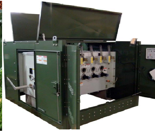
Figure 41: Pad-mounted SF6-Insulated Switch
