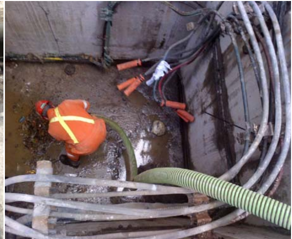
Figure 32: Crews Cleaning a Network Vault after a Network Transformer Leaked Oil
