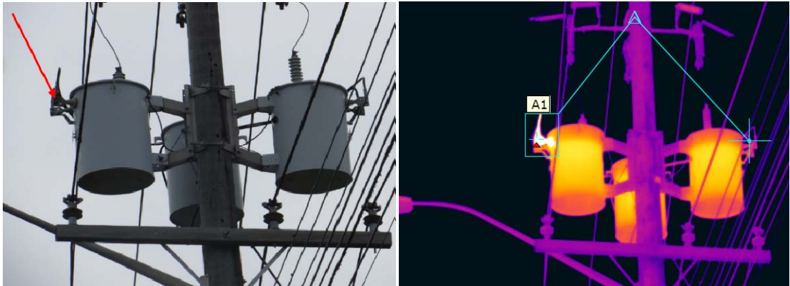
4 Figure 1: Secondary connection on pole-mounted transformer (Left) with an 5 infrared thermography image of the same asset denoting a hot spot at A1 (Right)
