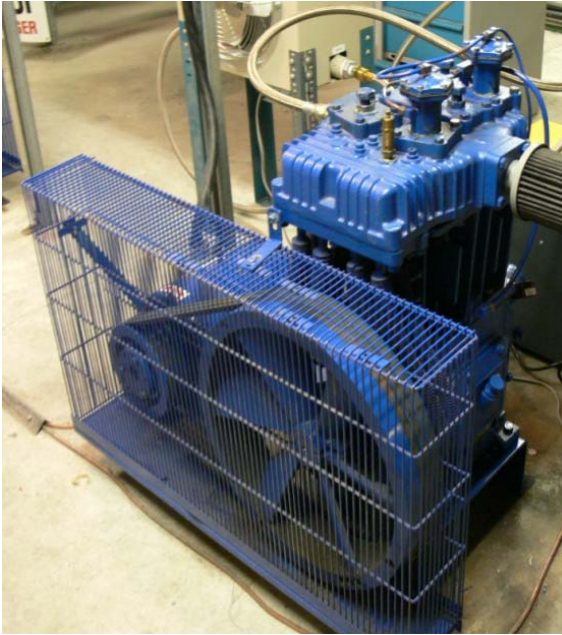
Figure 65: Air Compressor System
