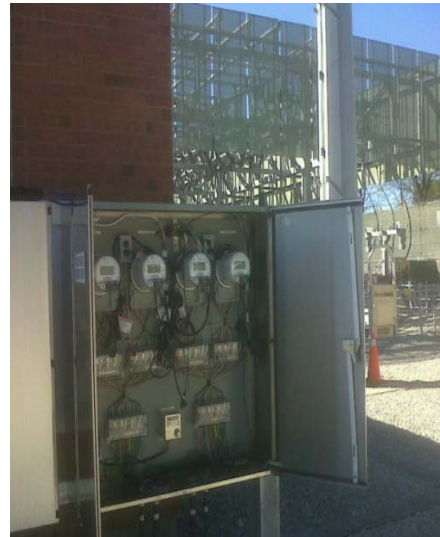
Figure 58: Wholesale meter installation at Transformer Station.
