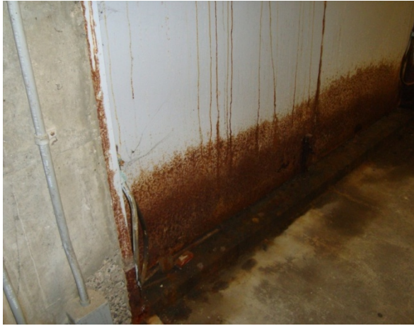
Figure 72: Rusty Switchgear Enclosure
