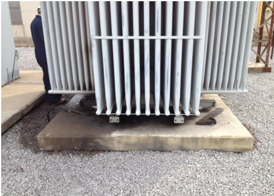
12 Figure 68: Oil Leak on a Station Transformer
