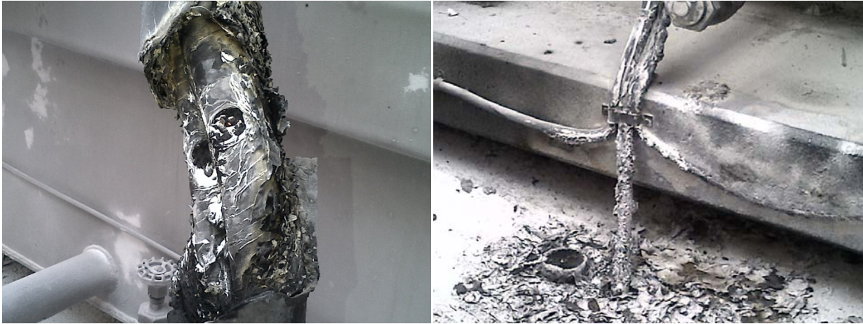
1 Figure 51: Aftermath of a cable failure resulting in a fire
