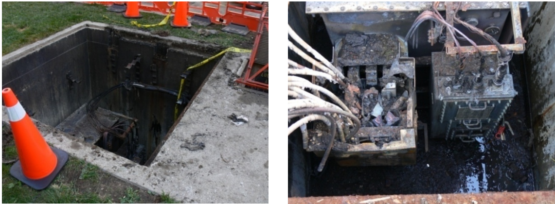
Figure 37: (Left) Vault 4557 with roof slabs off, signs of heavy smoke apparent in vault. (Right) damaged Fibertop Network Unit. (June 1, 2010)
