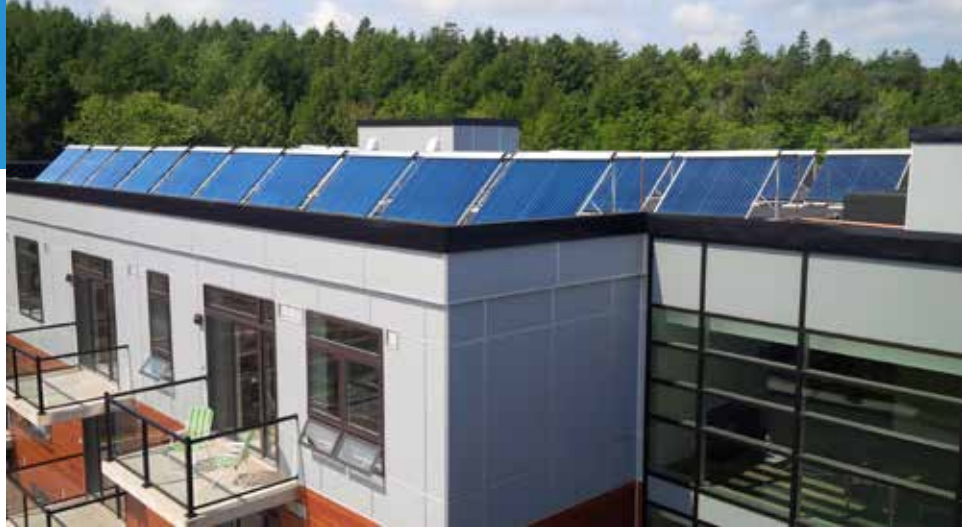
Apartment water heating, NS | Encom
