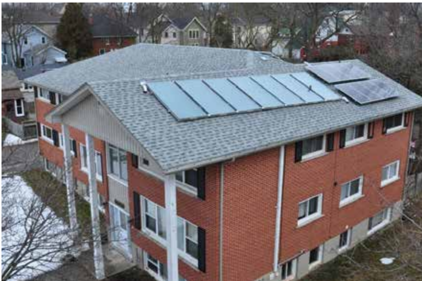
Apartment water heating, ON | Guelph Solar
