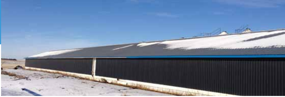
Chicken Barn air heating, AB | Solarwall
