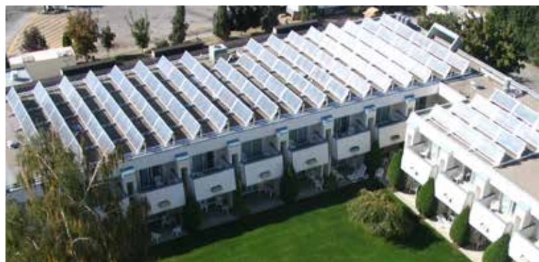
Hotel water heating, BC | Swiss Solar Tech
