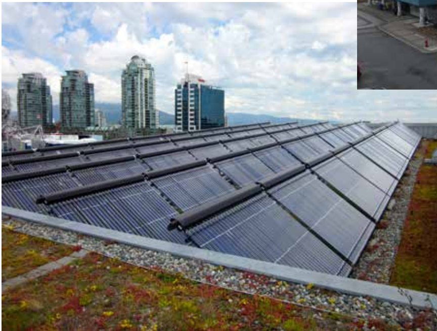
Commercial water heating, BC | Viessmann
