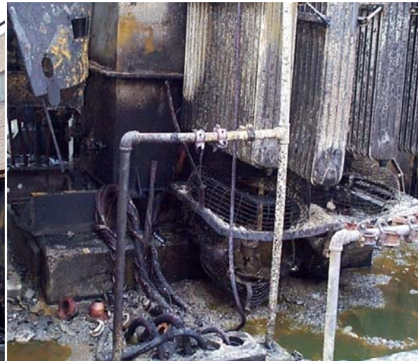
Figure 86: Leaking fluids from failed transformer
