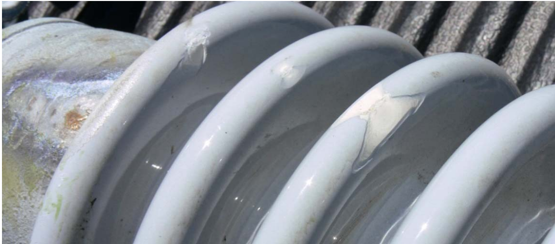
3 Figure 16: Close-up of Damaged Porcelain Insulator showing tracking
