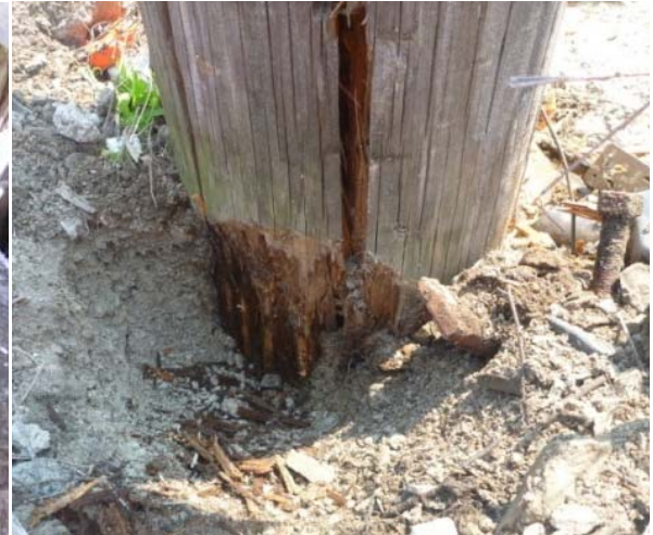
Figure 4: External rot at base of a pole
