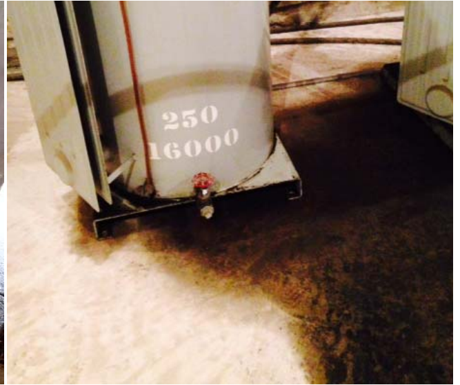
Figure 54: Transformer Leaking Oil
