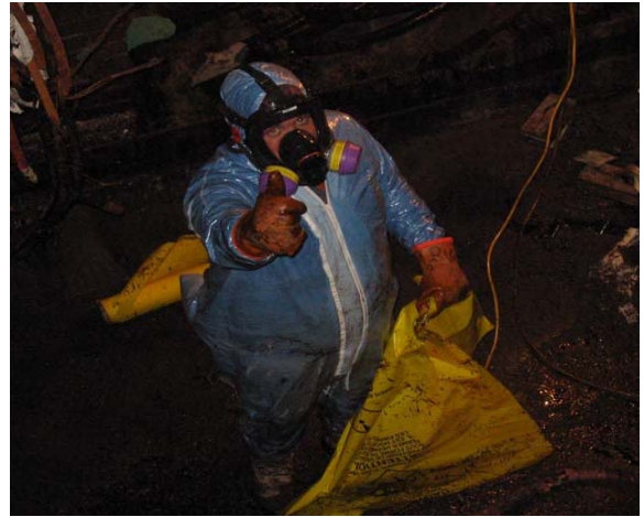
Figure 35: Asbestos clean after the fire.
