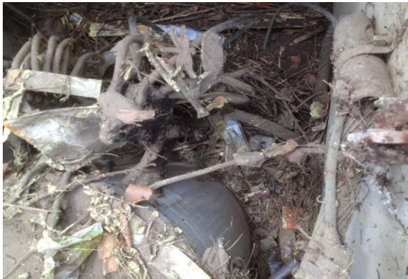
Figure 29: Vault full of Dirt and Debris
