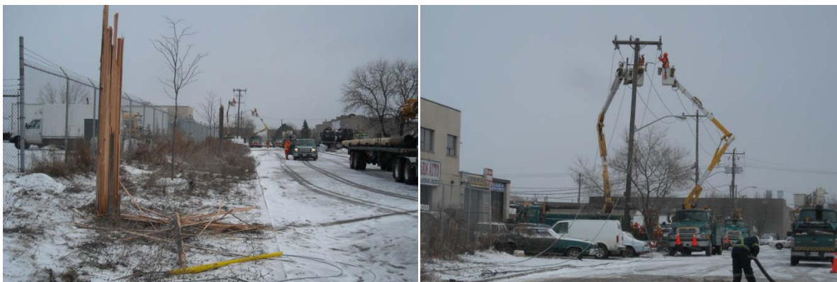
Figure 9: Damage caused during a storm on February 19, 2011.
