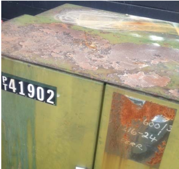
Figure 44: Pad-mounted Transformer with surface corrosion
