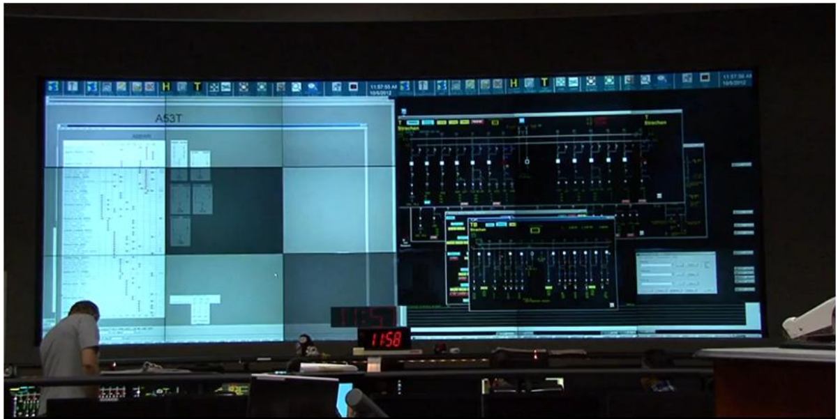
1 Figure 1: Toronto Hydro Control Room display and operating area.
