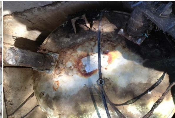
Figure 30: Corrosion on top of a Transformer
