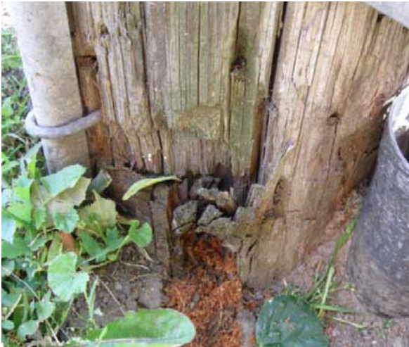
Figure 3: Internal rot at base of a pole
