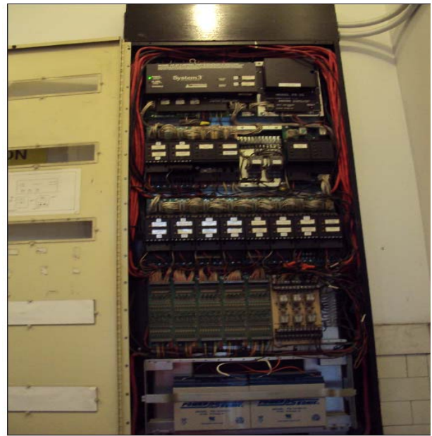
Figure 64: Fire Alarm Control Panel
