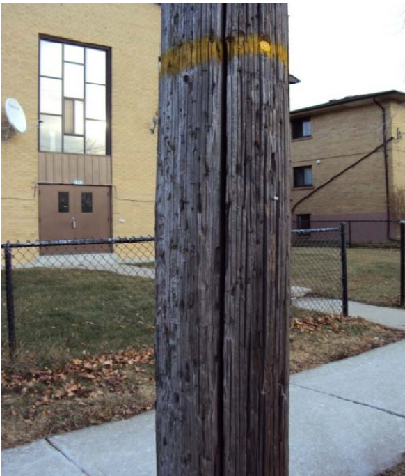
Figure 5 : Large crack along pole length
