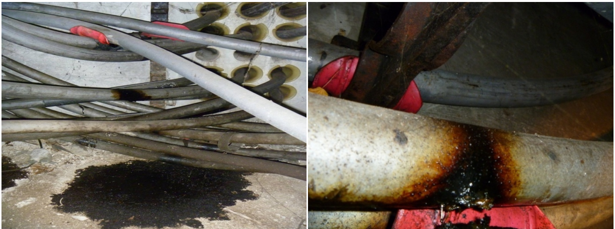
9 Figure 49: Oil Leakage from PILC Cable
