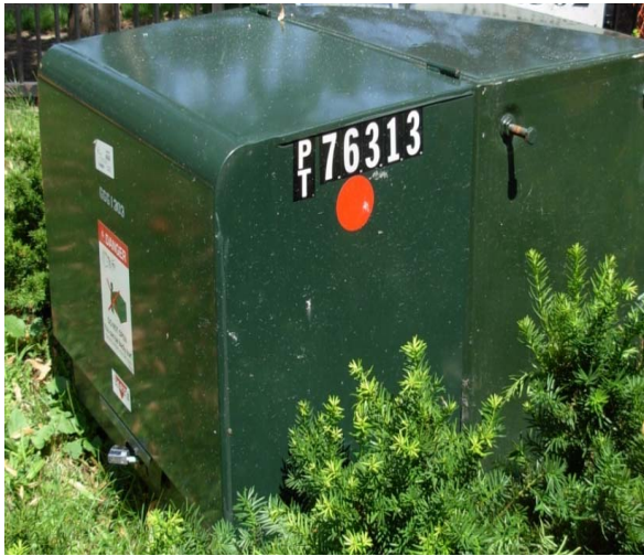
Figure 40: Pad-mounted Transformer in Residential Neighbourhood
