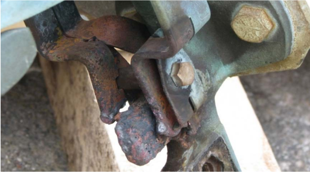
1 Figure 14: Corrosion of Switch Blade
