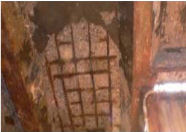
Figure 23: Vault Roof Exposed Rebar
