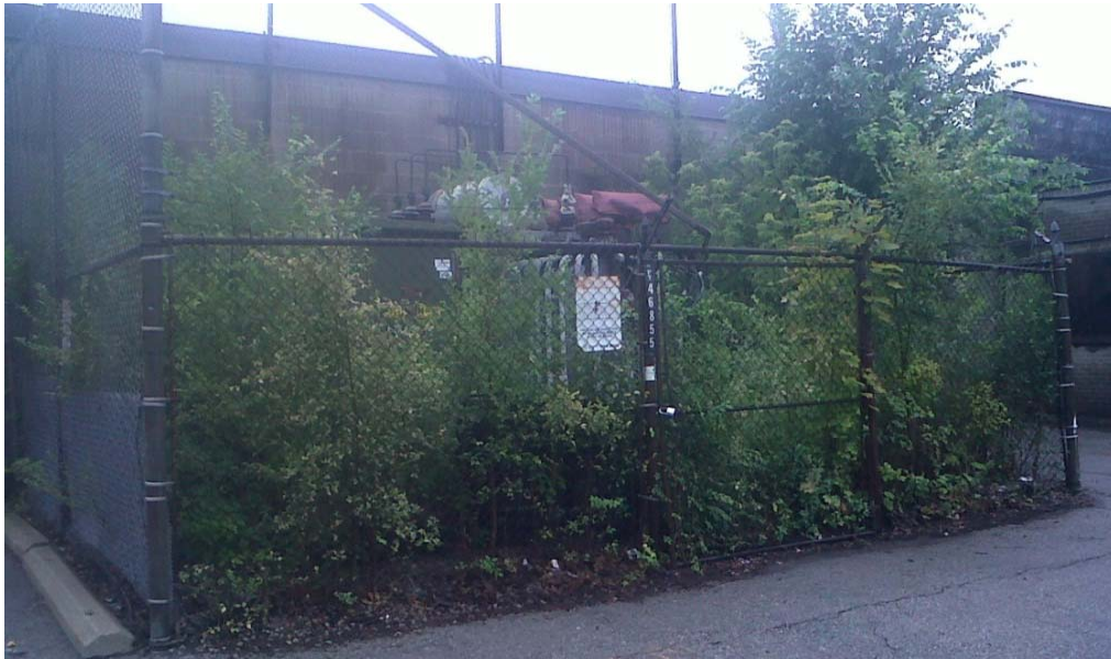
1 Figure 46: Pad-mounted Transformer requiring vegetation removal
