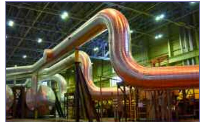
Steam lines in the Bruce B turbine hall.
