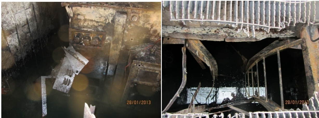
18 Figure 33: Damage from the 95 St. Clair Network Vault Fire
