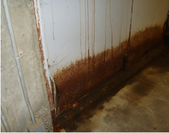
Figure 72: Rusty Switchgear Enclosure
