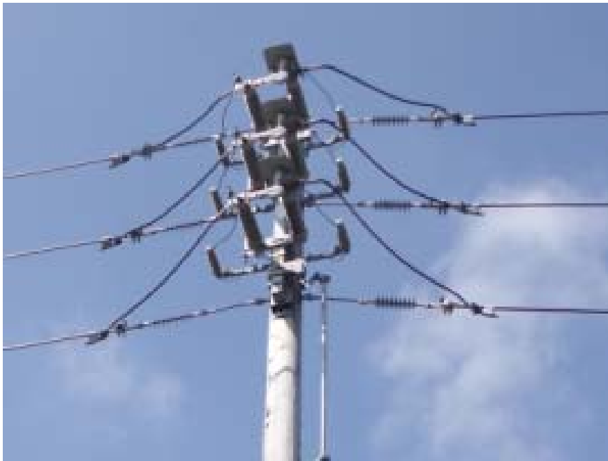
Figure 10: Manual Gang-Operated Switch
