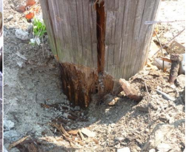
Figure 4: External rot at base of a pole
