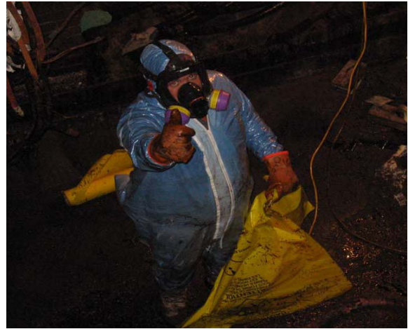
Figure 35: Asbestos clean after the fire.
