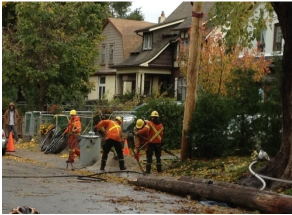
Figure 10: Damage caused during Hurricane Sandy on October 30, 2012.
