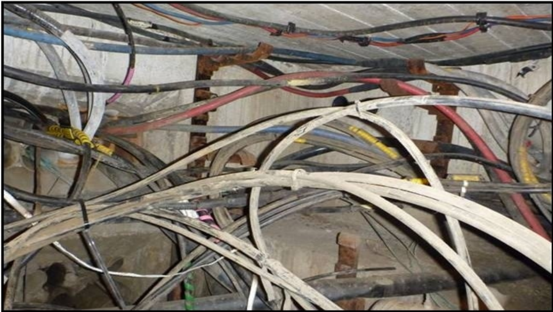
4 Figure 4: Underground cable chamber in Toronto Hydro's system.
