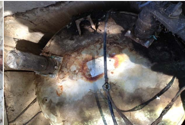
Figure 30: Corrosion on top of a Transformer
