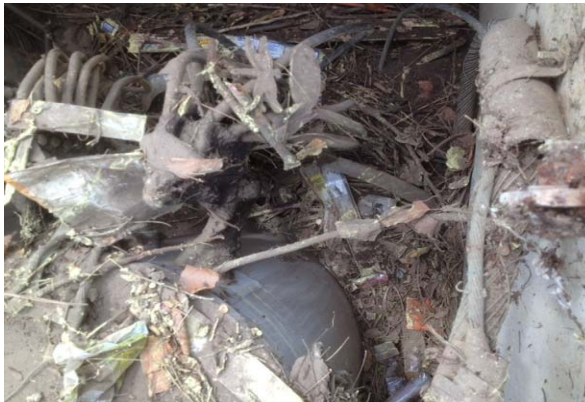
Figure 29: Vault full of Dirt and Debris
