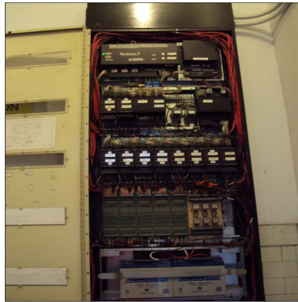
Figure 64: Fire Alarm Control Panel
