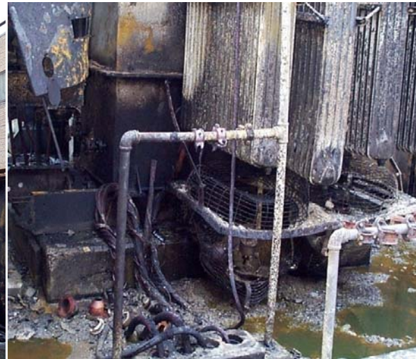
Figure 86: Leaking fluids from failed transformer
