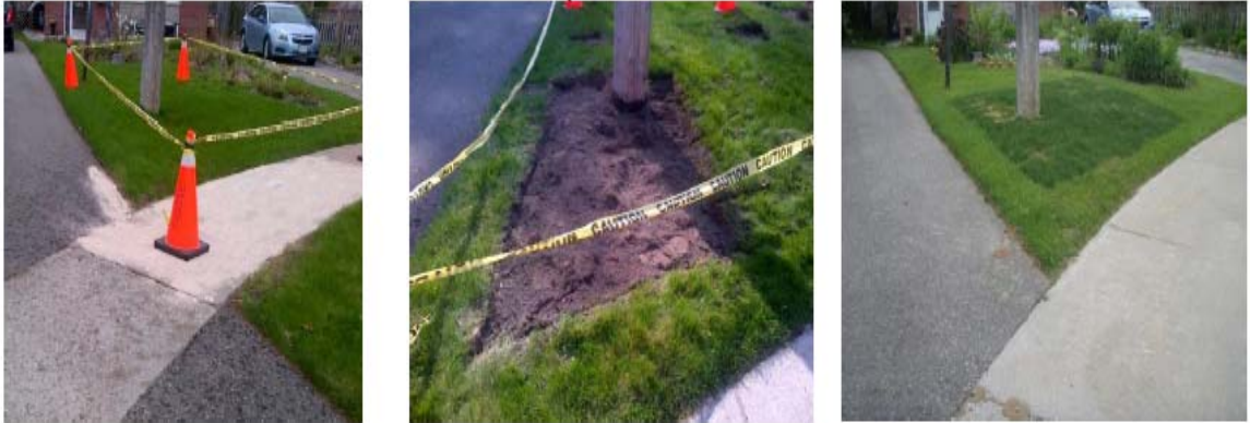
1 Figure 8: Response to a leaking transformer in a residential area. Response 2 pictures are before, during, and after remediation work undertaken by a Grid 3 Response crew.
