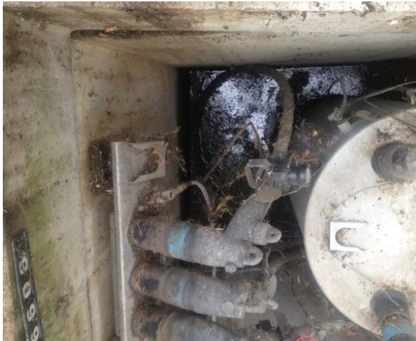
Figure 31: Oil Leak at the bottom of the Transformer
