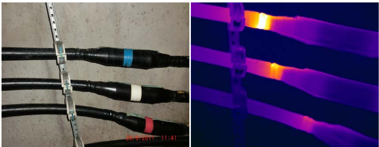
Figure 39: Cables inside a cable chamber (left) with a with a thermographic image of the same (right)
