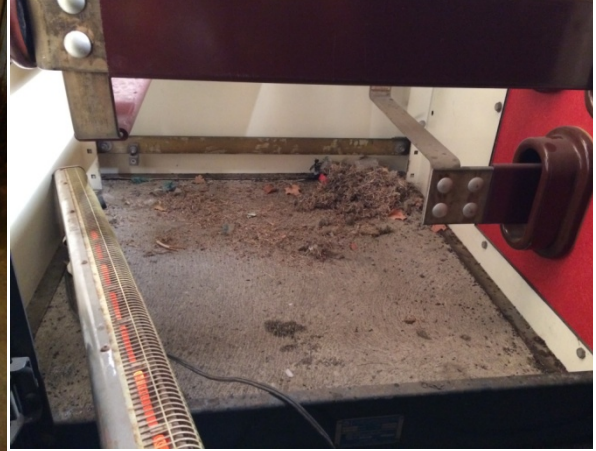
Figure 73: Pests inside Outdoor Switchgear
