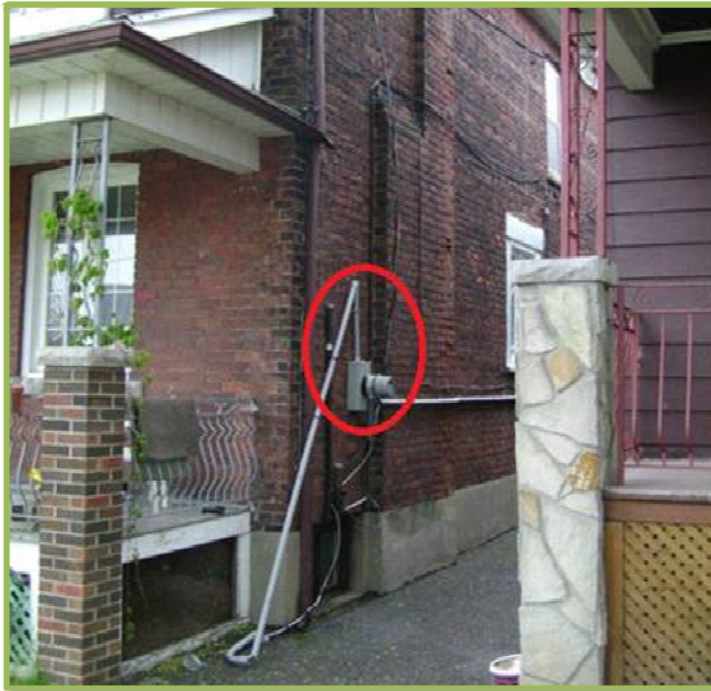
Figure 14: Example of Mast Damage
