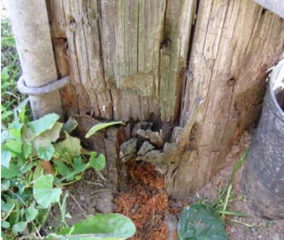
Figure 3: Internal rot at base of a pole
