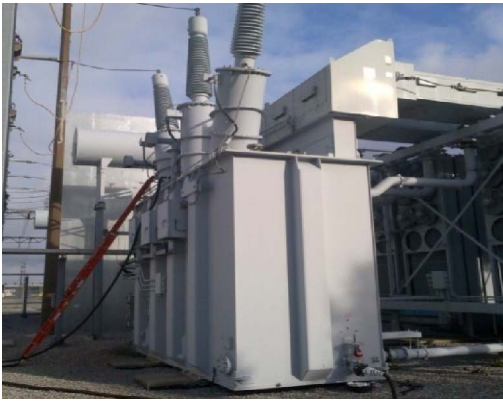
Figure 81: Power Transformer at Cavanagh TS
