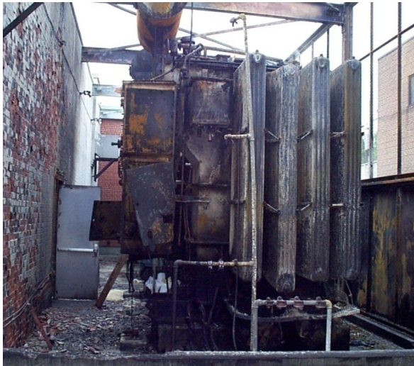
Figure 85: Damages to the MS wall on the Left
