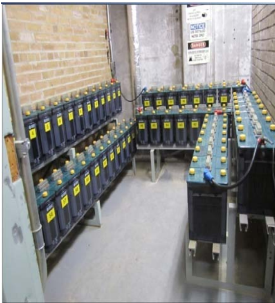
Figure 63: Station Battery System at George and Duke MS
