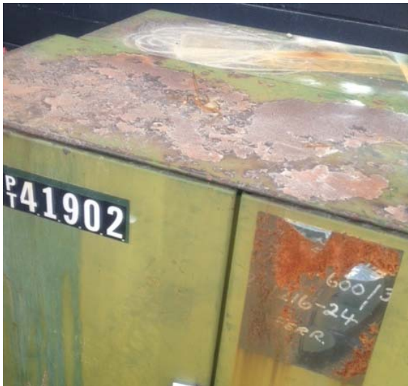
Figure 44: Pad-mounted Transformer with surface corrosion
