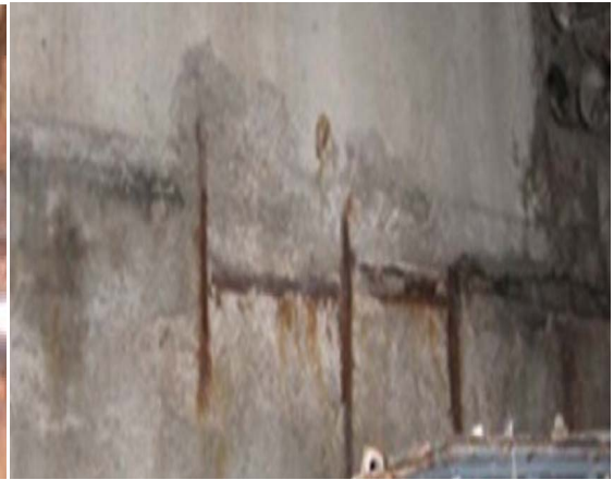
Figure 24: Vault Wall Exposed Rebar
