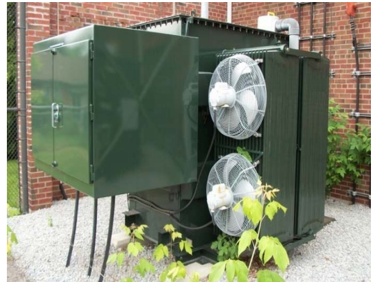
Figure 82: Power Transformer at Neilson Dr. MS
