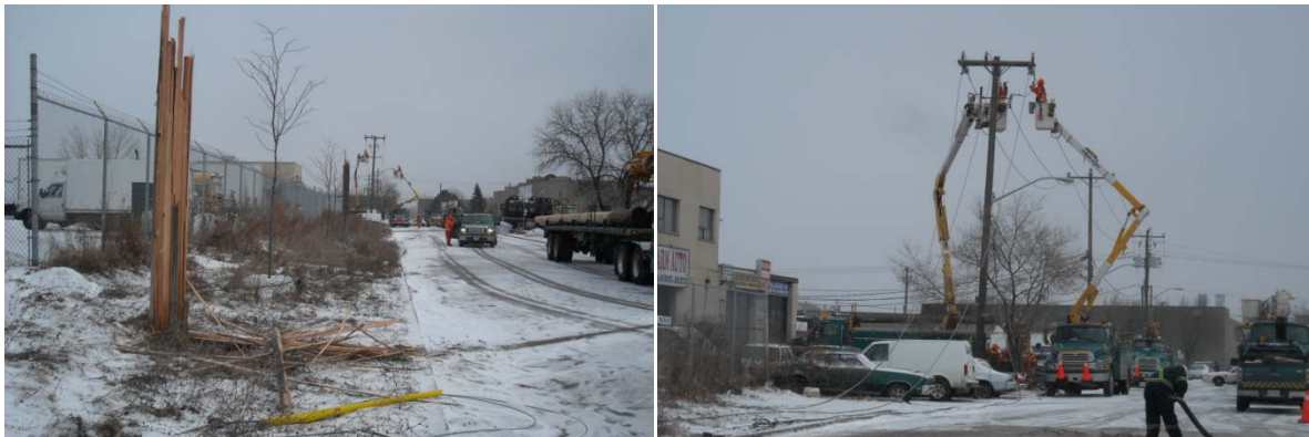
Figure 9: Damage caused during a storm on February 19, 2011.
