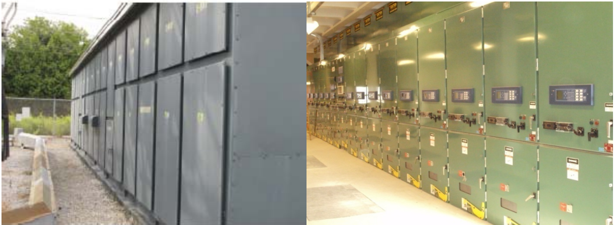
Figure 70: (Left) Outdoor Enclosure Housing Metalclad Switchgear. (Right) Indoor Metalclad Switchgear
