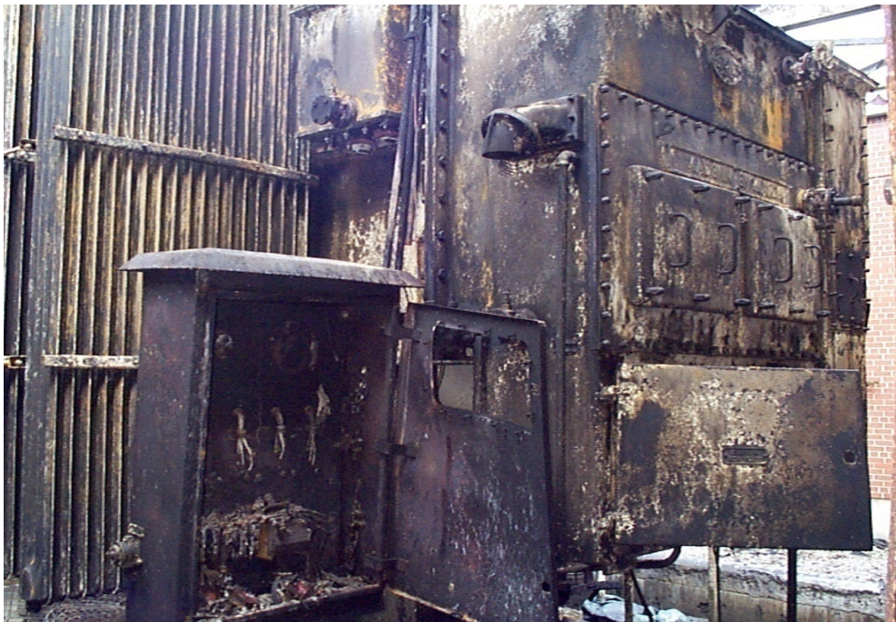
5 Figure 84: Failed Power Transformer
