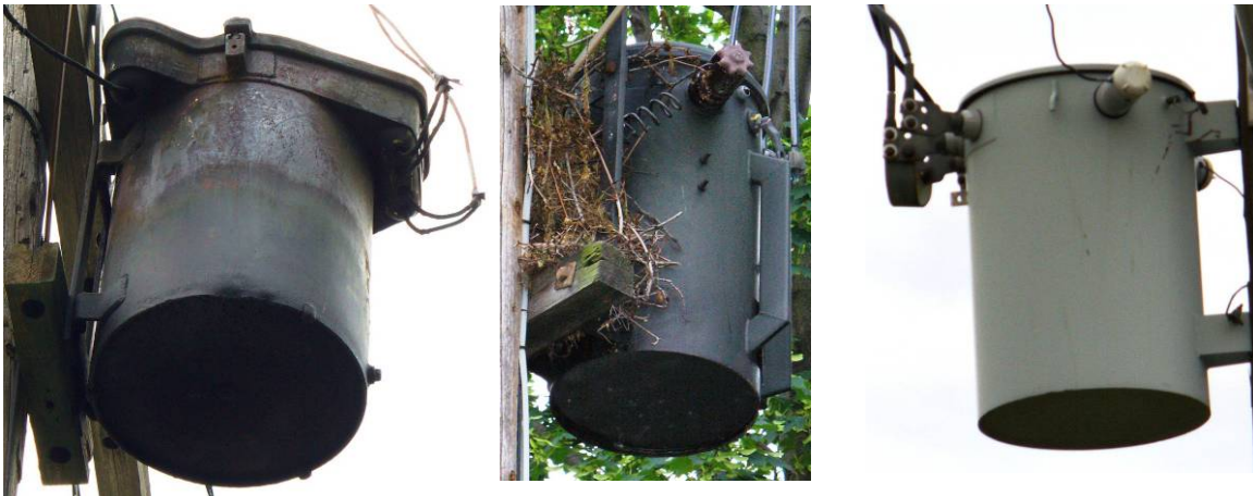
Figure 4-30 Example Pole Mounted Transformers
