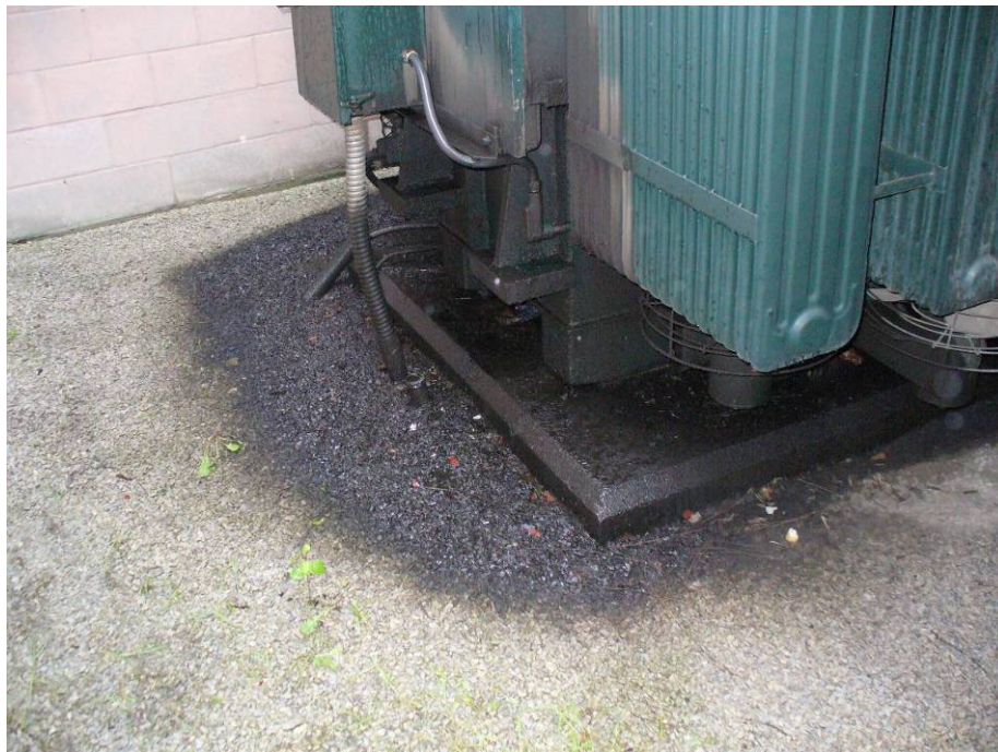
Figure 4-10 Example 27.6kV -13.8kV Power Transformer
