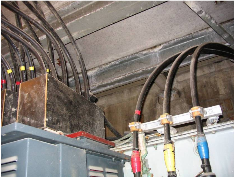
Figure 4-40 Example Network Vault
