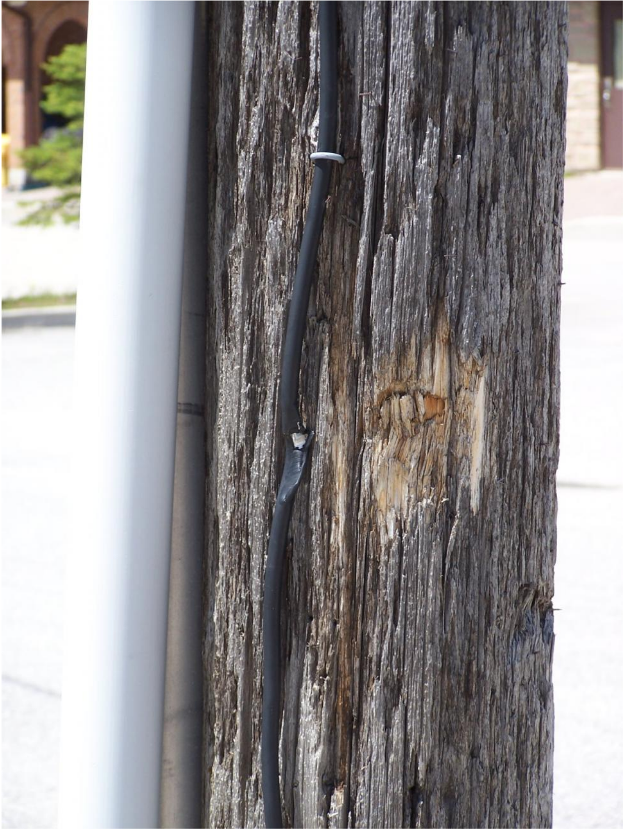
An example of wood deterioration
