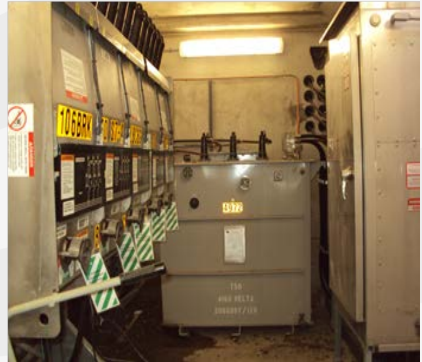
New Submersible Transformer, Gas Switchgear and Secondary Breaker Panel
