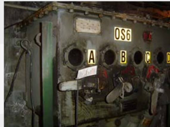
End-of-Life Oil Insulated Switchgear
