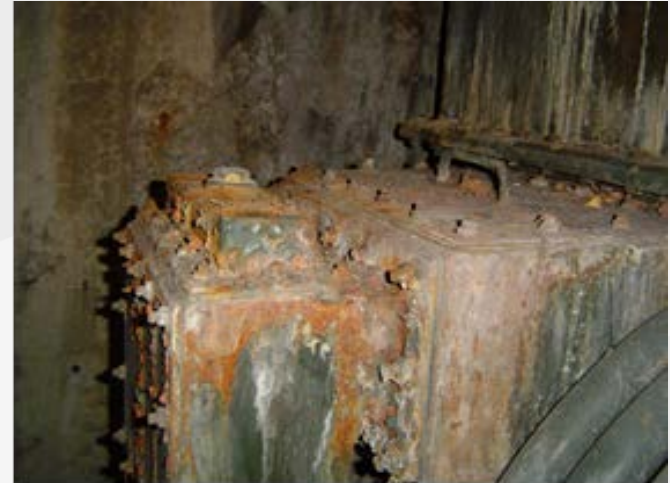
End-of-Life Submersible Transformer
