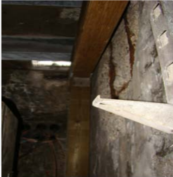
Exposed and Corroded Wall
