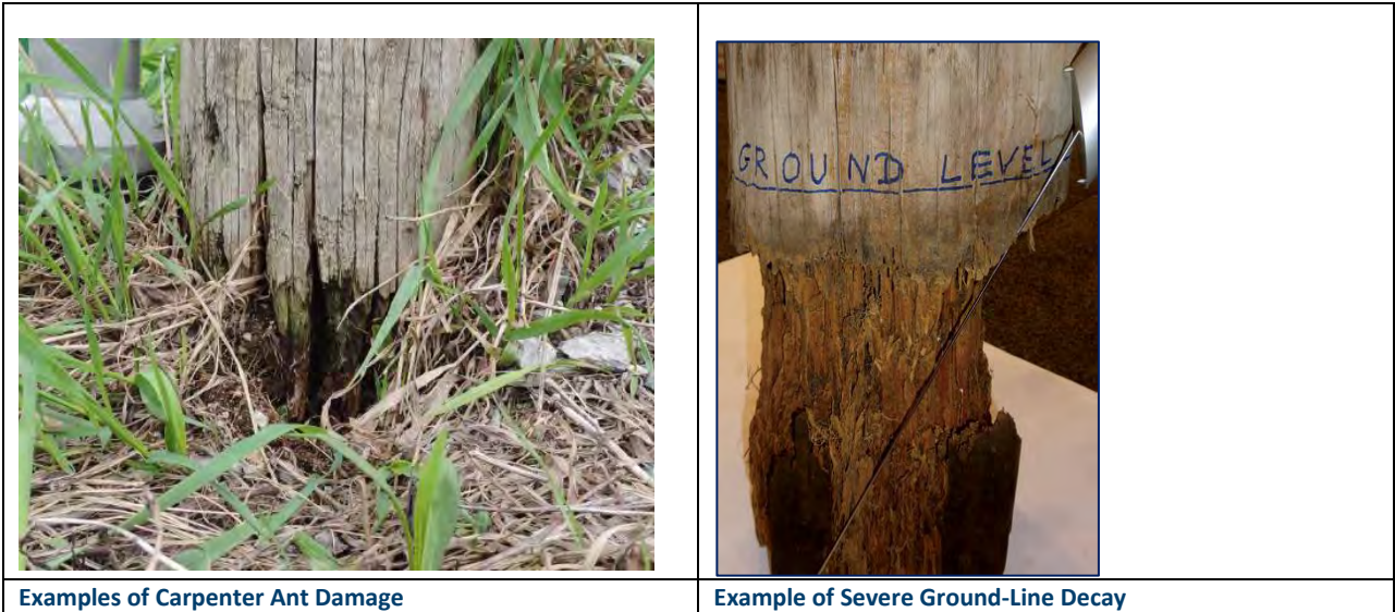
Figure 19 Examples of Pole Damage
