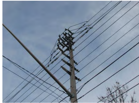
Figure 25 46kV Loadbreak Switch
