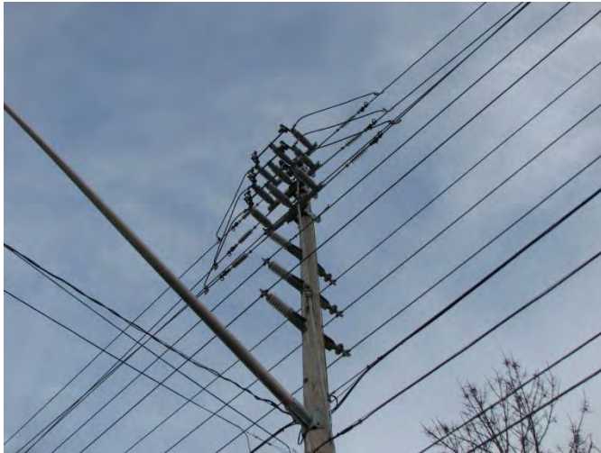
Figure 52 46kV Loadbreak Switch
