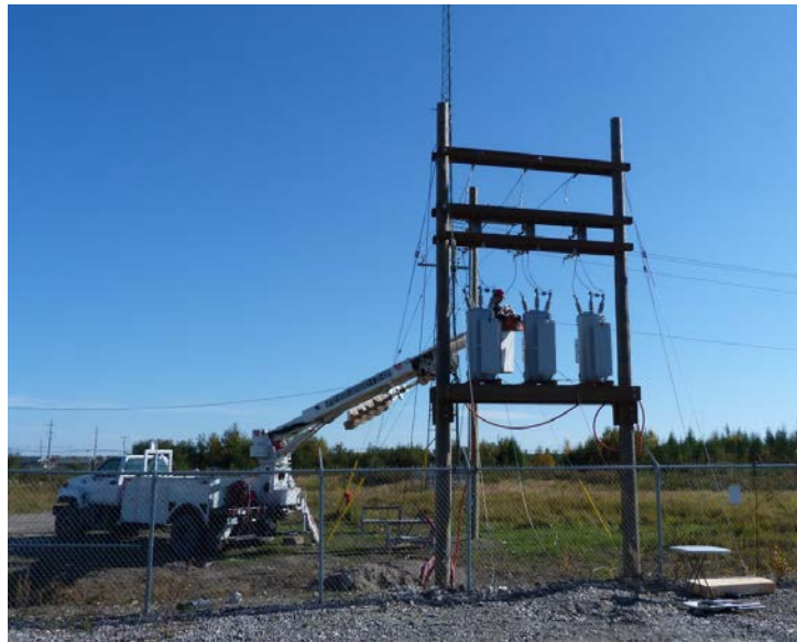
Kashechewan connection point (regulators shown)
