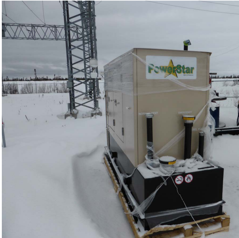
Back-up generator prior to installation in Kashechewan
