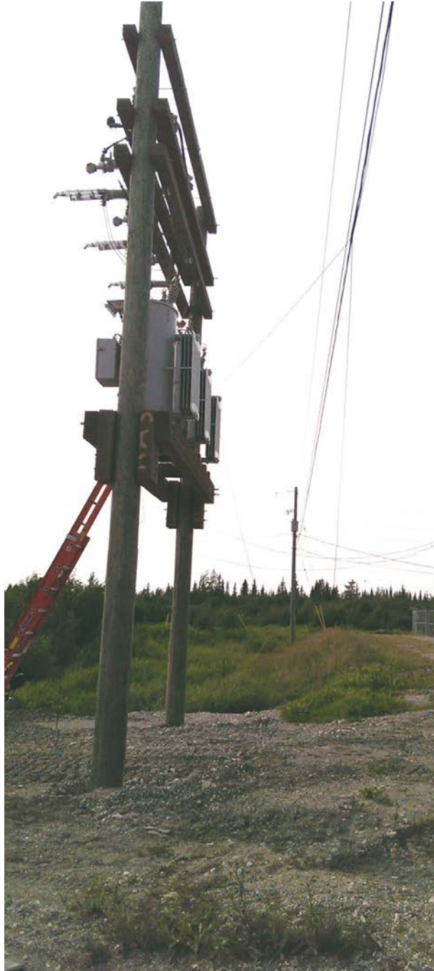
Attawapiskat connection point (regulators shown)
