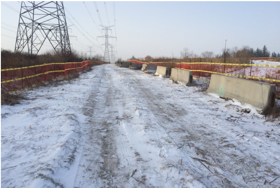
Photo 18 – Jersey barriers and snow fencing installed to stop construction activities through the Pengilley Archaeological Site (January 2015)
