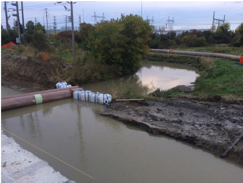
Photo 16 – Some stormwater overwhelming the cofferdam at Spring Creek (September 2015)
