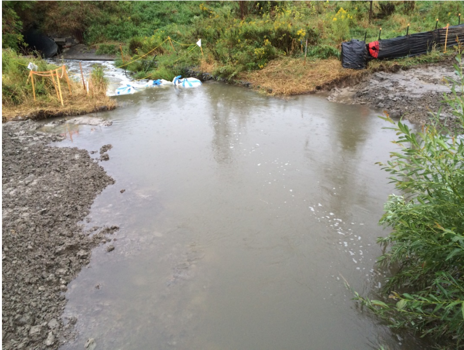
Photo 17 – Stormwater overwhelming the worksite prior to final restoration of the channel for the isolated open-cut of German Mills Creek (September 2015)
