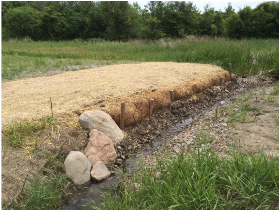
Photo 14 – Mullet Creek in June 2016 after addressing some minor bank erosion (June 2016)
