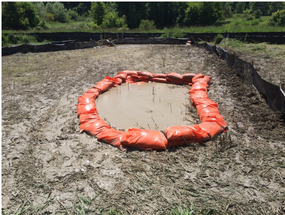
Photo 4 – Segregating IFR from watercourse using sand bags and sediment fence in a layered approach at the East Don River (July 2015)
