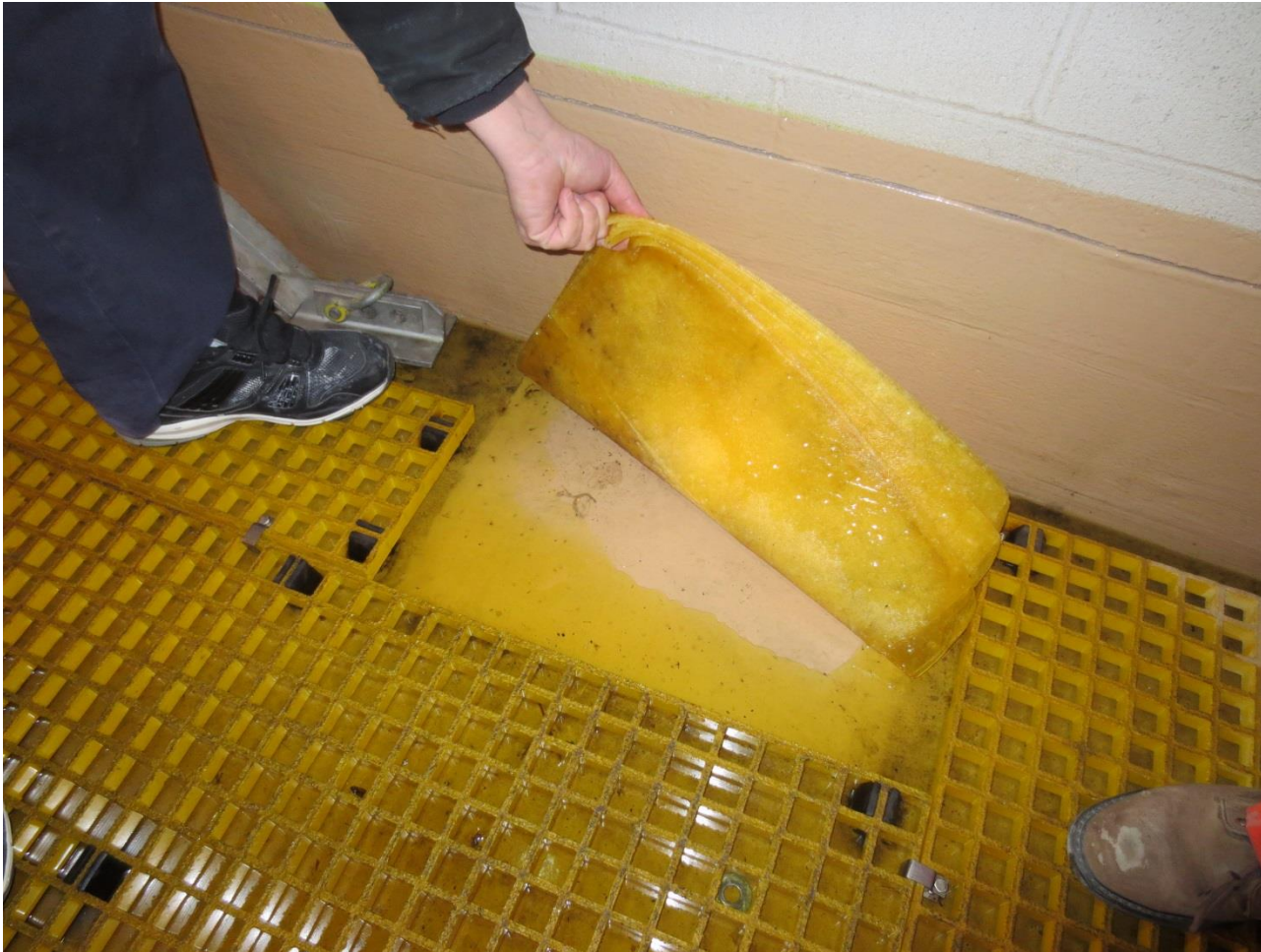
Picture of T1's bay showing puddles of oil accumulated on the ground (Picture taken 2015 Q1)
