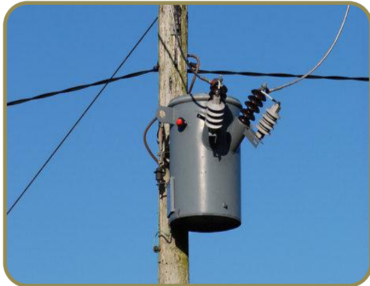
Pole Mounted Transformer
