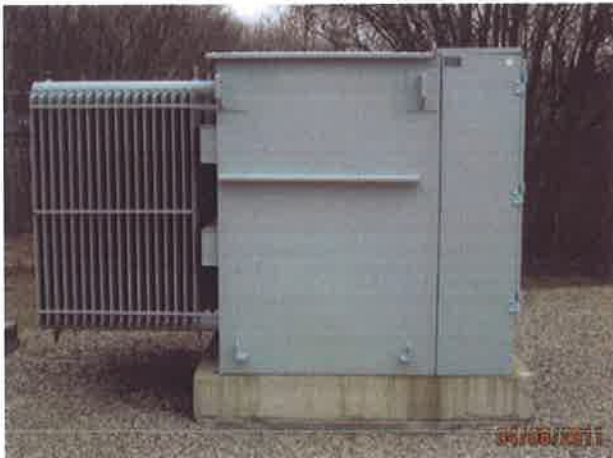
New Padmount Transformer
