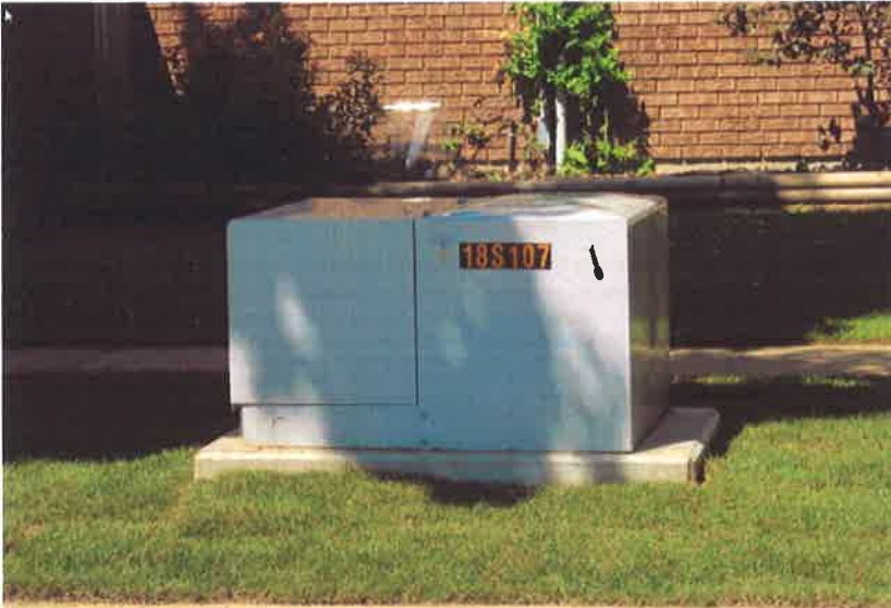
New Padmount Transformer
