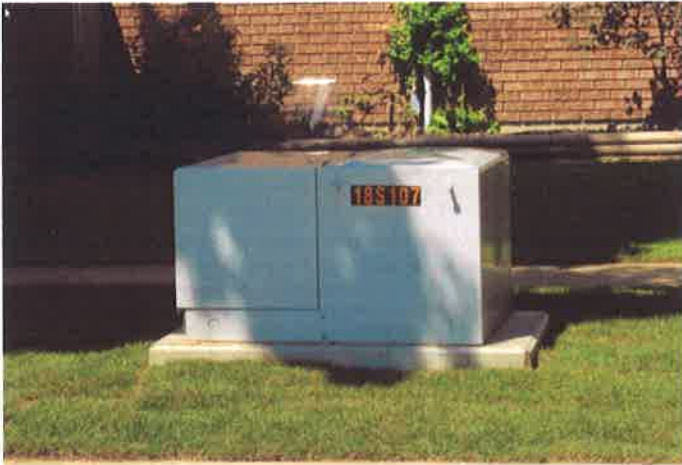
New Padmount Transformer
