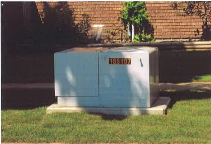
New Padmount Transformer
