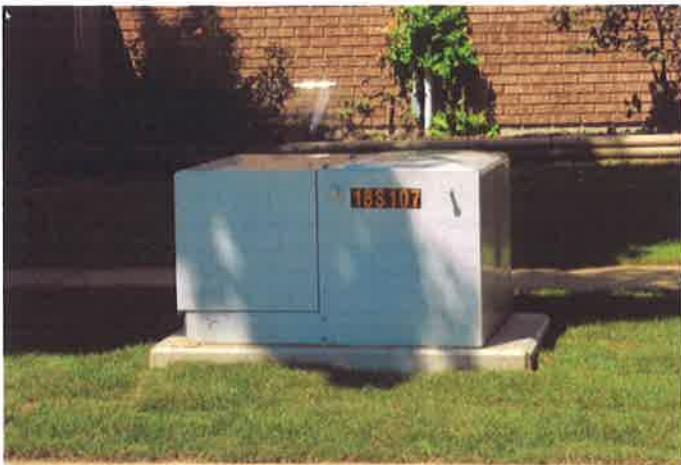
New Padmount Transformer
