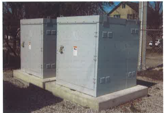
New Sectionalizer Reclosers
