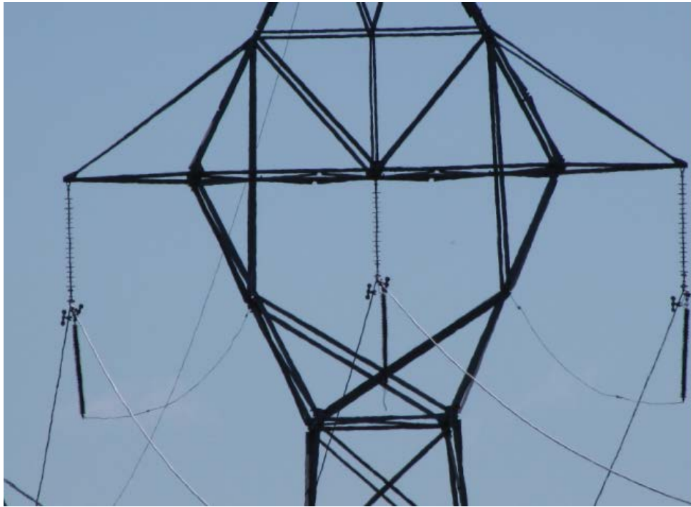
Figure 12-8 - Surge Arrester Connected Bond Wire (A1B, structure 2, 115 kV)
