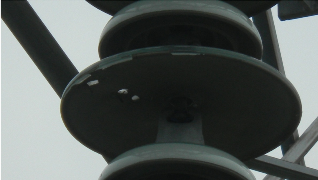
Figure 11-2 - Silicone on Glass Insulator
