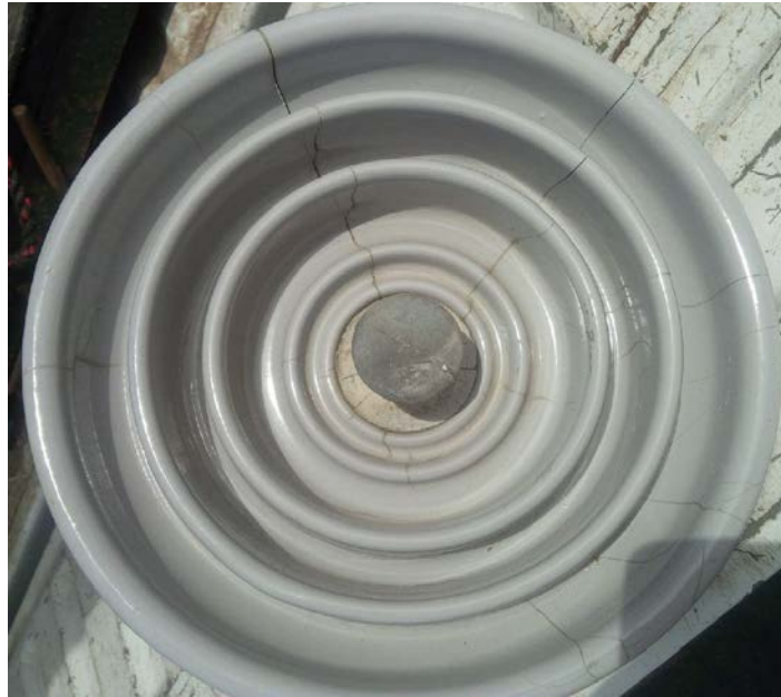
Figure 8-2 - Porcelain Insulator Unit Affected by Cement Expansion (V79R, Structure 50E, April-2015)
