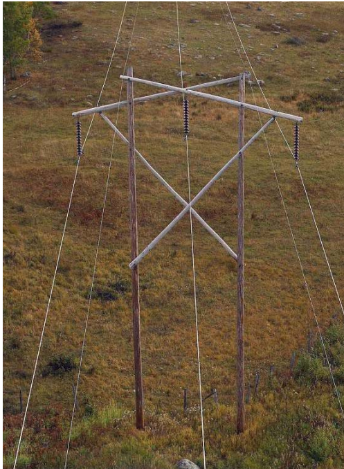
Figure 7-1 – I-Suspension (K23D, structure 4, 230 kV, porcelain)
