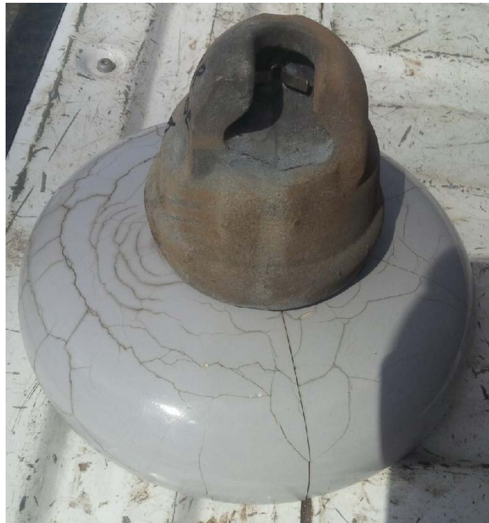
Figure 8-1 - Porcelain Insulator Unit Affected by Cement Expansion (V79R, Structure 50E, April-2015)
