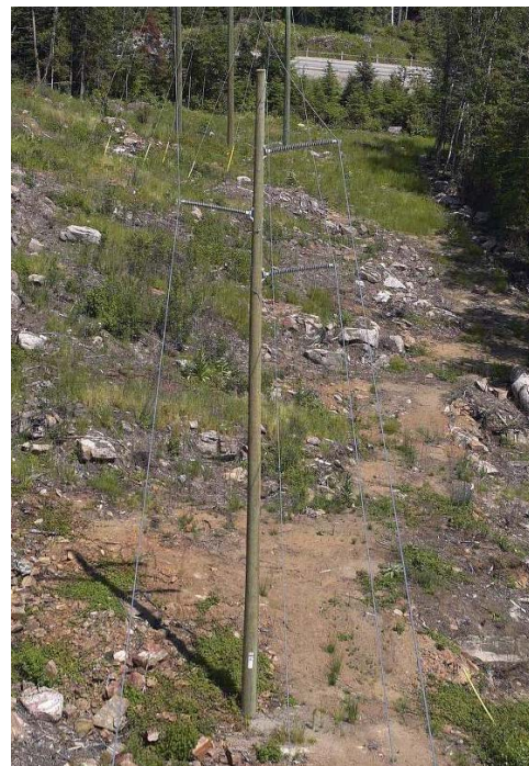
Figure 7-4 – Post (L5H, structure 444A, 115 kV, polymer)
