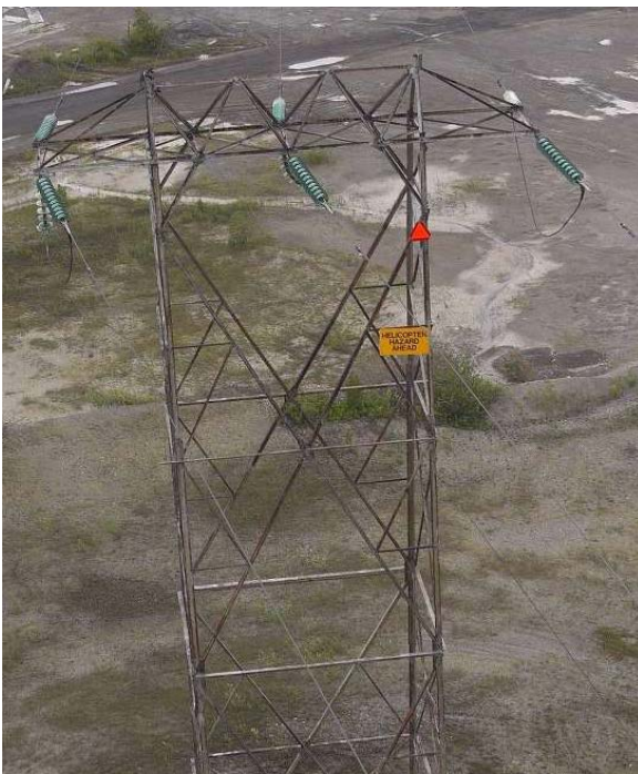
Figure 7-3 – Dead-end with Idler (C1P, structure 34, 115 kV, glass)
