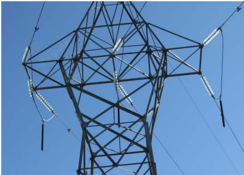
Figure 12-9 - Surge Arrester Disconnected Bond Wire (A1B, structure 1, 115 kV)
