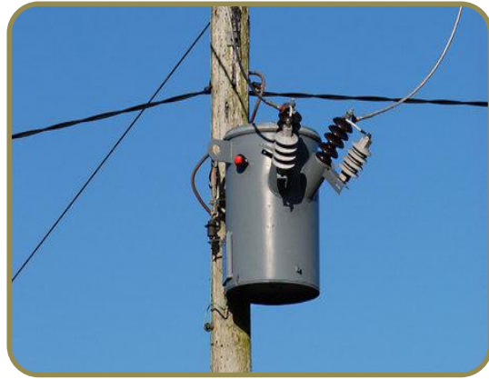
Pole Mounted Transformer
