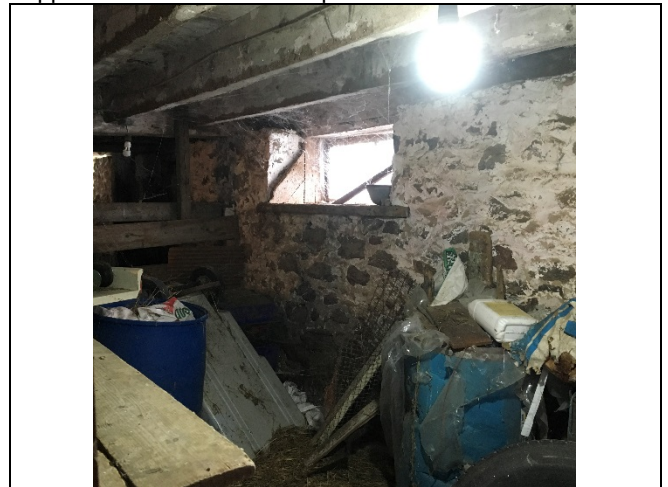
Photo 22: The east foundation wall appears to be similar to the pre-construction assessment.
