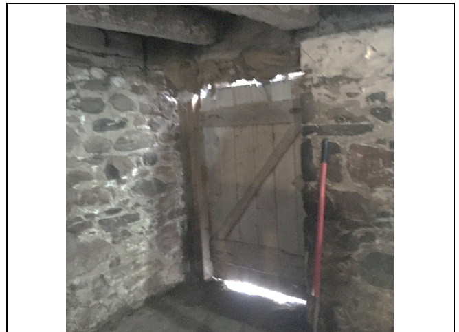
Photo 18: The condition of the basement door access appears to be similar to the pre-construction assessment.
