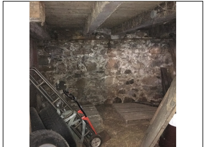
Photo 12: No apparent change to the west foundation wall
