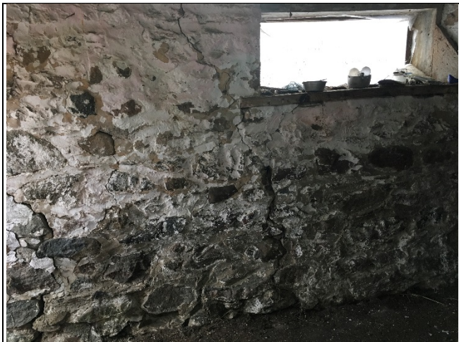
Photo 3: E2 – View of crack on south foundation wall in the basement
