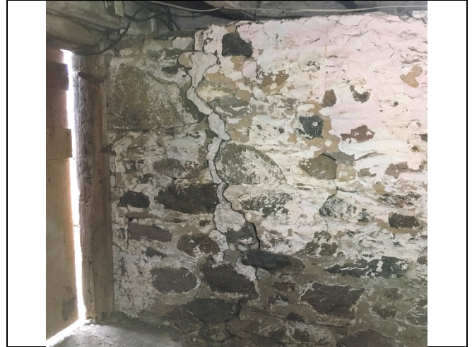
Photo 2: No significant change to the crack on the south foundation wall was observed.
