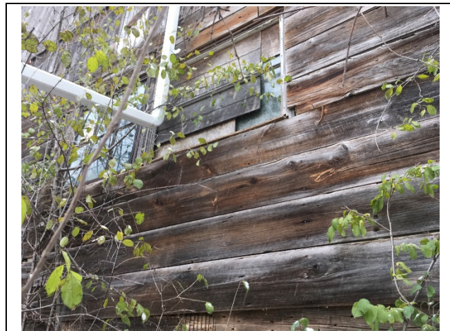
Photo 41: E21 – View of the boarded damaged window and damaged wood boards on the south elevation
