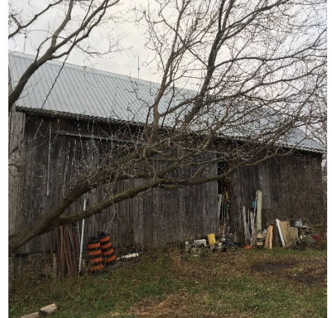
Photo 58: The condition of the west elevation appears to be similar to the pre-construction assessment.
