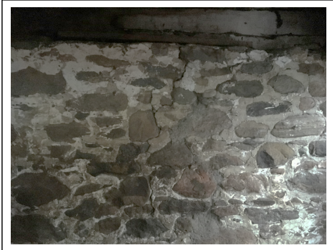
Photo 15: E8 – View of a crack on the north foundation wall
