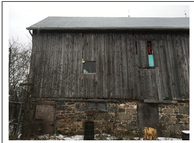
Photo 51: E26 – View of the damaged wood boards on the east elevation
