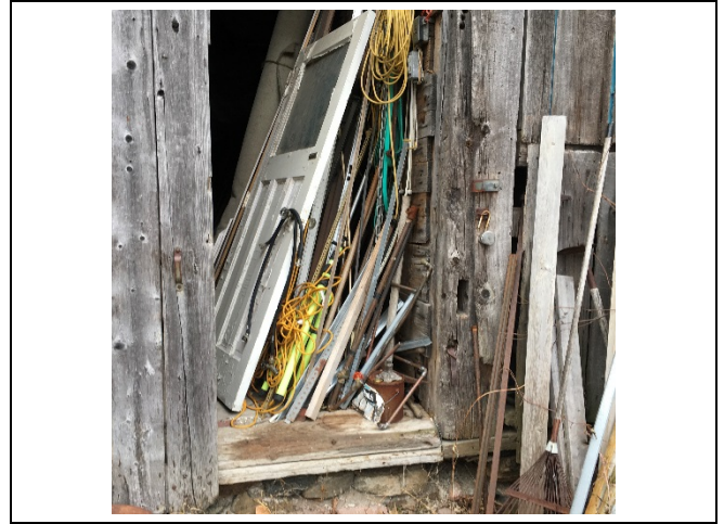
Photo 64: The condition of the lower portion of the sliding door appears to be consistent with the pre-construction initial assessment.
