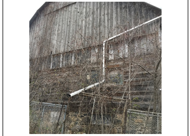
Photo 50: On the south elevation, no significant change to the damaged wood boards was observed.
