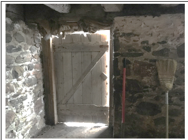
Photo 17: E9 – On the east elevation,- a view of the basement door access
