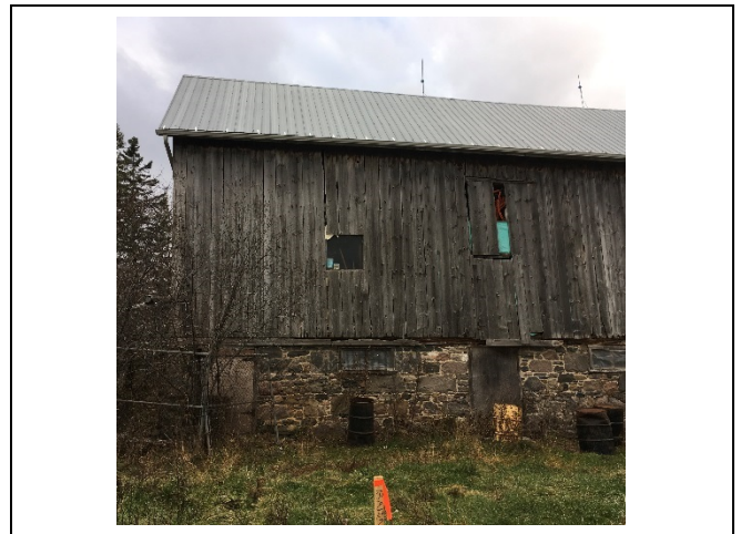
Photo 52: No significant change to the damaged wood boards was observed on the east elevation
