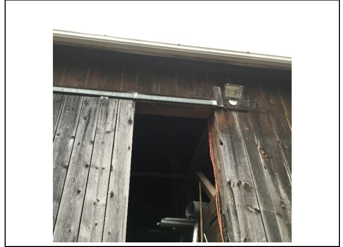
Photo 62: The condition of the wood boards above the sliding door appears unchanged.
