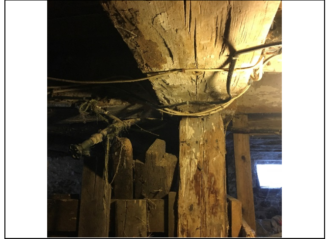
Photo 32: The wood post and floor joist appear to be consistent with the pre-construction assessment.
