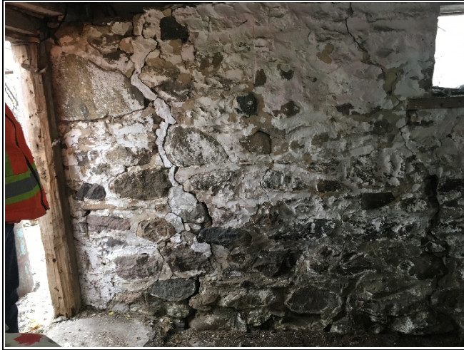
Photo 1: E1 – View of a crack on south foundation wall in the basement
