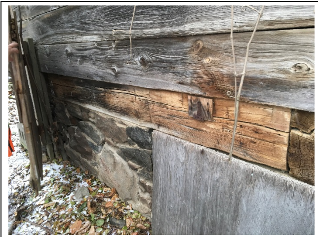
Photo 45: E23 – View of the damaged wood boards on the south elevation
