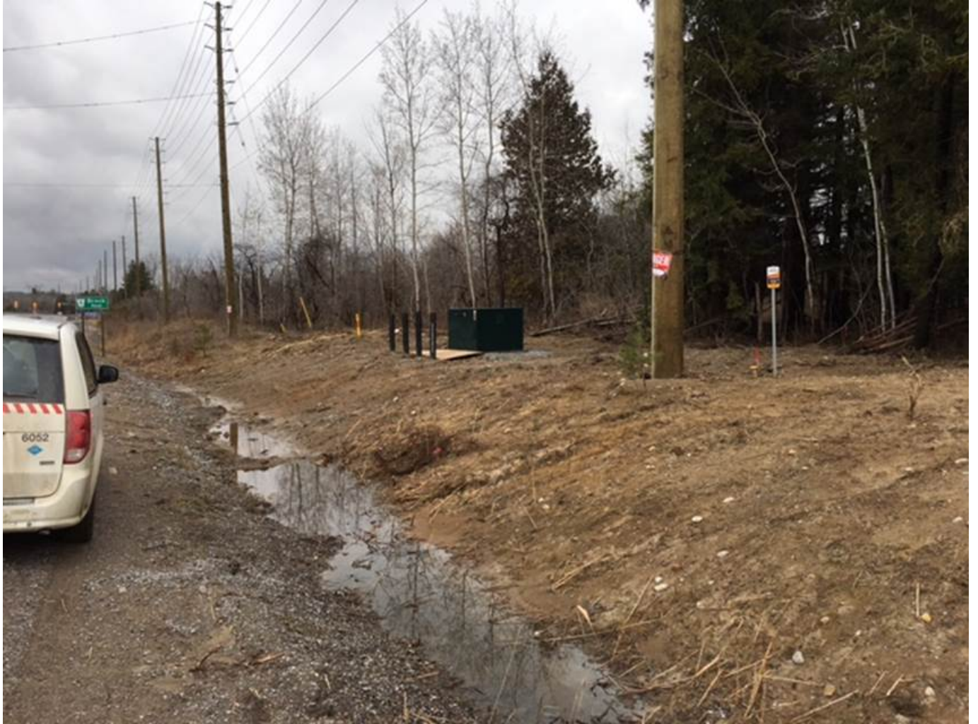
Photo 3: Regulator Station east of Brock Rd (looking north-west)
