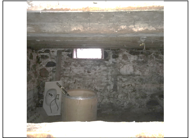
Photo 8: No significant change to the condition of the west foundation wall was observed following the construction.
