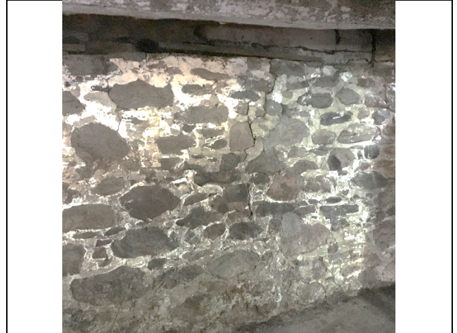
Photo 16: No significant change to the (north foundation wall) crack was observed.
