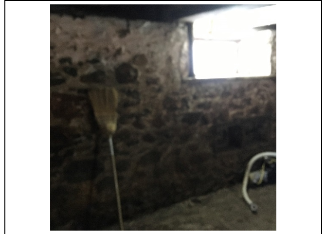
Photo 20: The condition of the east foundation wall appears consistent with the pre-construction assessment.
