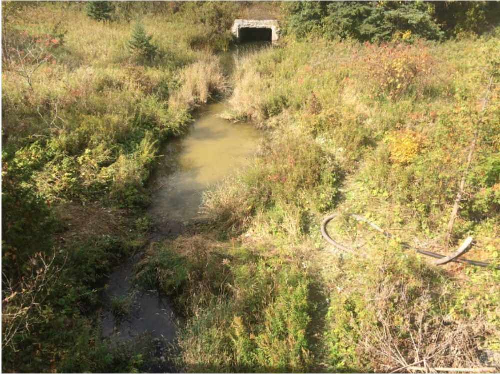
Photo 2: Condition of Urfe Creek on October 14, 2016 after the meeting with the MNRF and the TRCA
