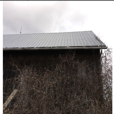
Photo 60: No significant change to the damaged wood boards was observed on the west elevation.
