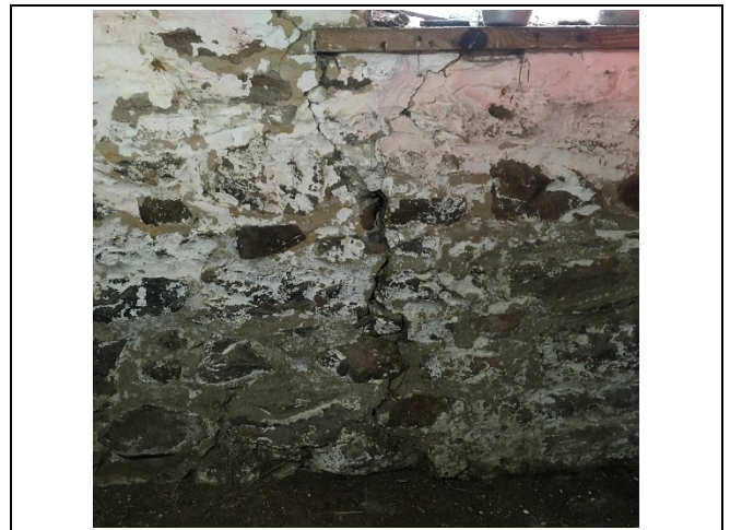
Photo 4: No significant change to the crack on the south foundation wall was observed.
