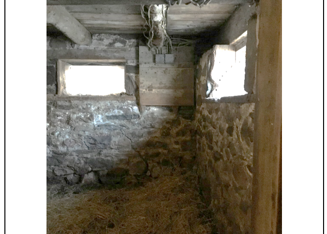
Photo 14: No significant change to the crack on the west foundation wall was observed.
