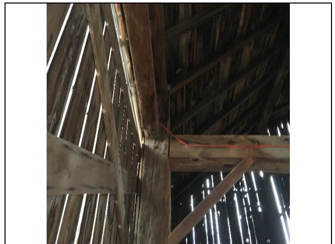
Photo 36: The condition of the wood roof frame structure appears to be consistent with the pre-construction assessment.
