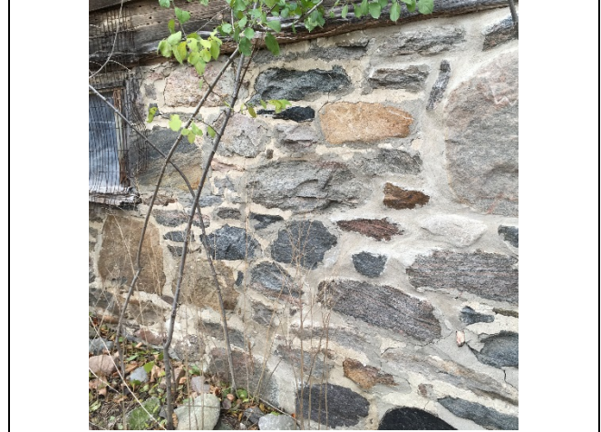
Photo 26: The south foundation wall appears to be similar with the pre-construction assessment.
