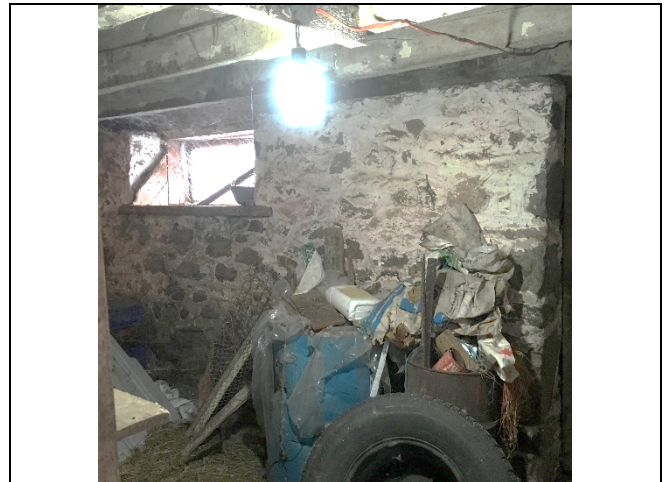
Photo 24: The east foundation wall appears to be consistent with the pre-construction assessment.
