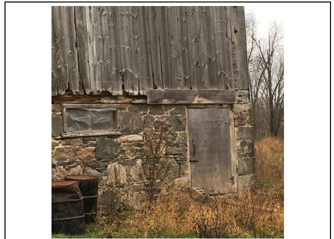
Photo 54: No significant change to the damaged wood boards was observed on the east elevation.
