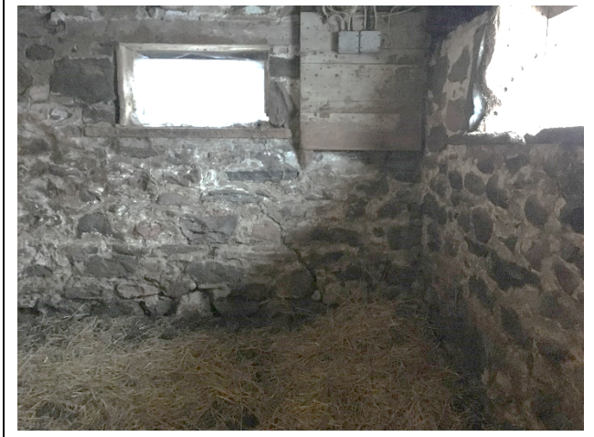
Photo 13: E7 –View of a crack on the west foundation wall (Animal Stable # 3)
