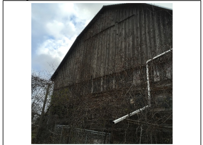
Photo 48: In general, the condition of the south elevation appears to be consistent with the pre-construction assessment.
