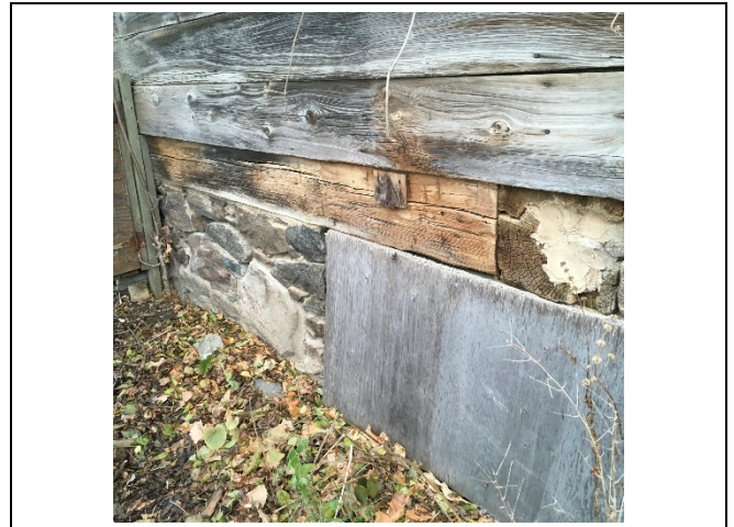
Photo 46: No significant change to the south elevation damaged wood boards was observed.
