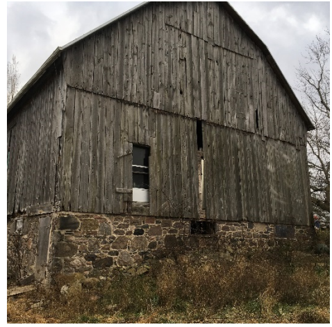
Photo 56: On the north elevation no significant change to the damaged wood boards was observed.
