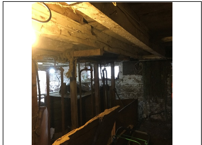
Photo 30: The condition of the floor joists appear to be similar to the pre-construction assessment.
