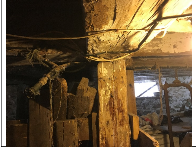
Photo 31: E16 – View of the wood post and floor joist in the basement
