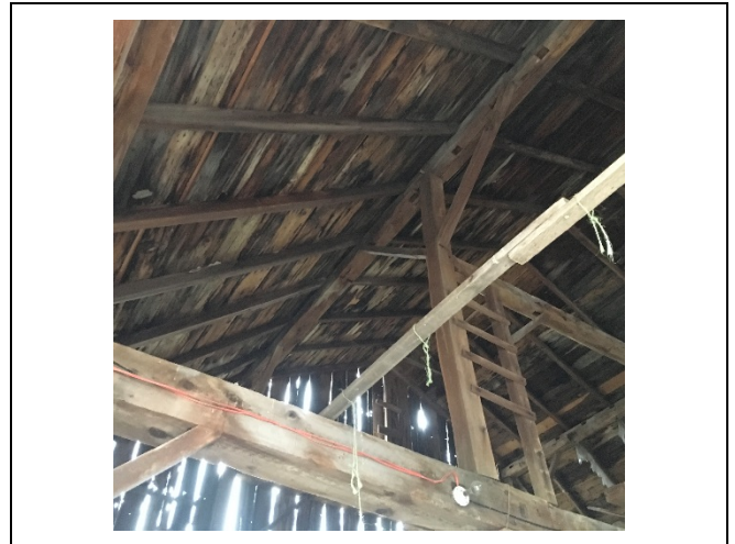
Photo 34: The first floor wood roof frame structure appears to be consistent with the pre-construction assessment
