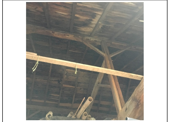
Photo 38: The condition of the wood roof frame structure appears to be similar with the initial assessment.
