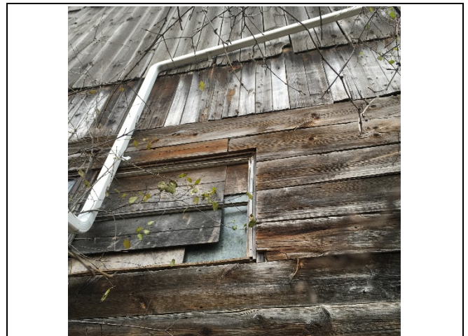
Photo 42: No significant change to the condition of damaged window and wood boards was observed.
