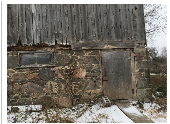
Photo 53: E27 – Closer view of the damaged wood boards on the east elevation
