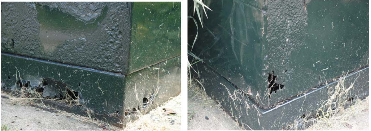
Figure 30: Excessive Corrosion of Enclosures on UG Pads
