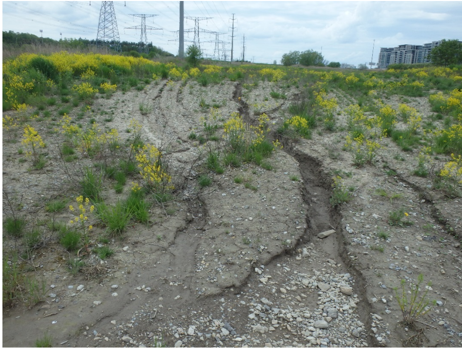
Photo 9 – Rills and gullies requiring remediation between Little German Mills and German Mills Creek, Site #1A (May 2017)
