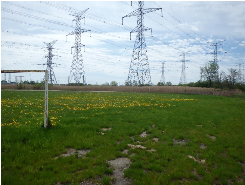
Photo 25 – Soccer field with subsidence requiring restoration to address subsidence on the ROW (May 2017)
