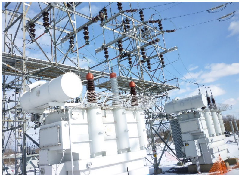
Figure 3: Existing (Original) Substation Transformers
