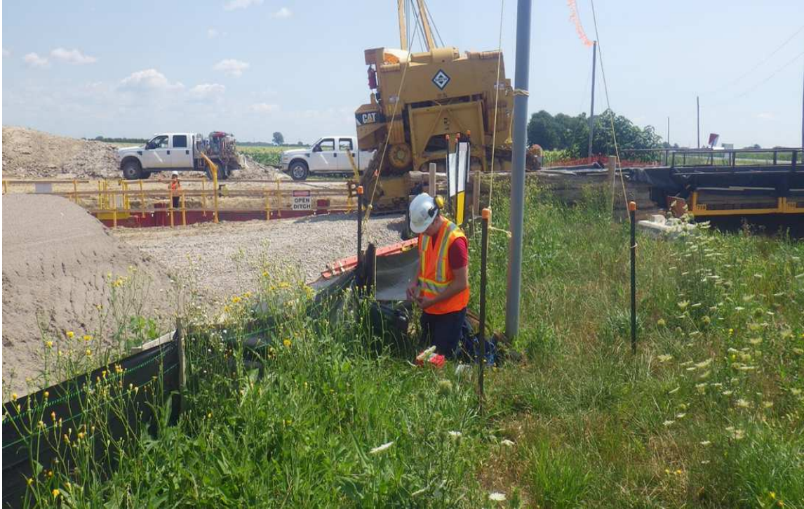
Stantec technician downloading vibration monitor at the Hwy 40 bore site. Completed as part of the MOECC Permit to Take Water.
