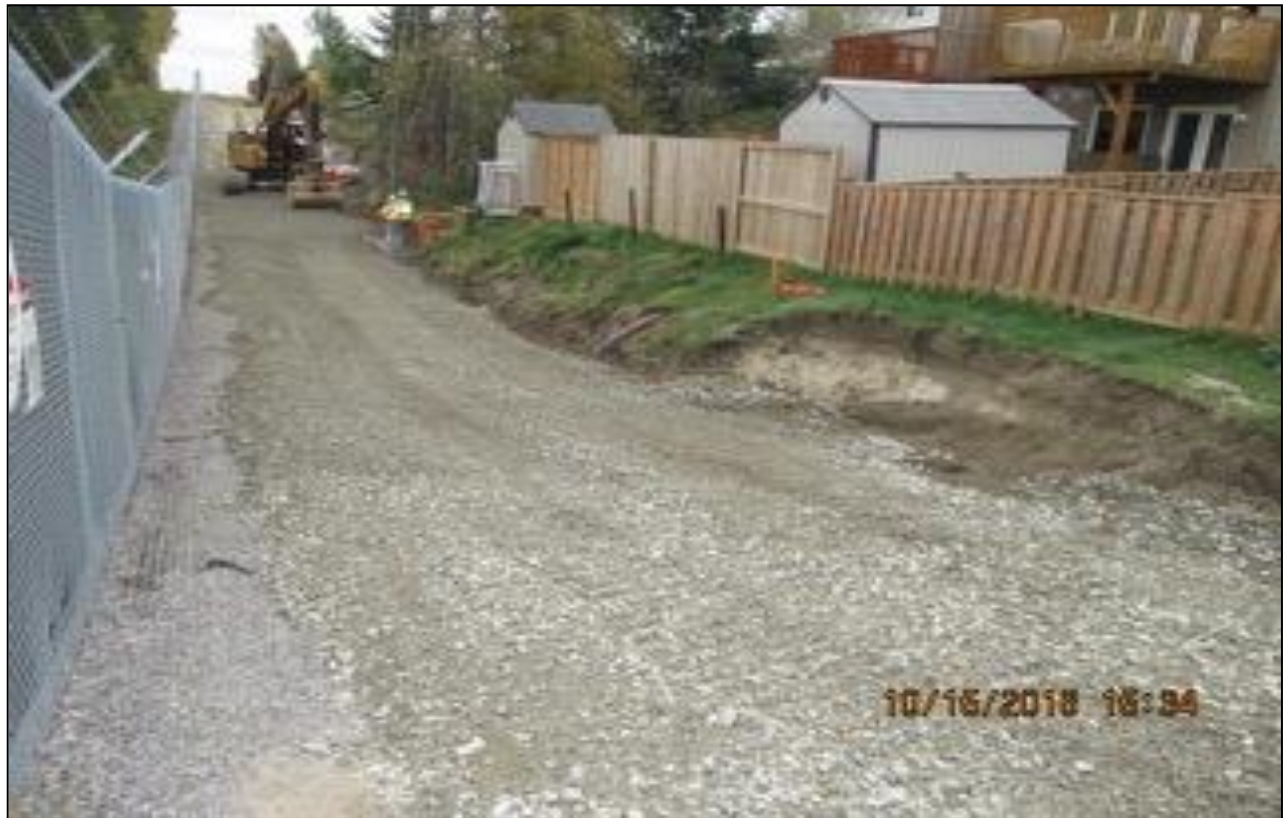
A portion of Section 1 construction was located between the fence of a Hydro One facility and private properties.
