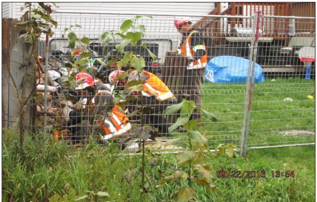
Safety fencing was installed along private yards that were open to the construction easement.
