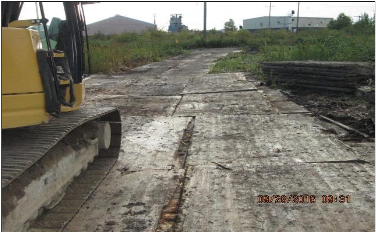
In areas of wet or unstable soils, large wooded mats are placed together to create a stable access with little disturbance to the soils.
