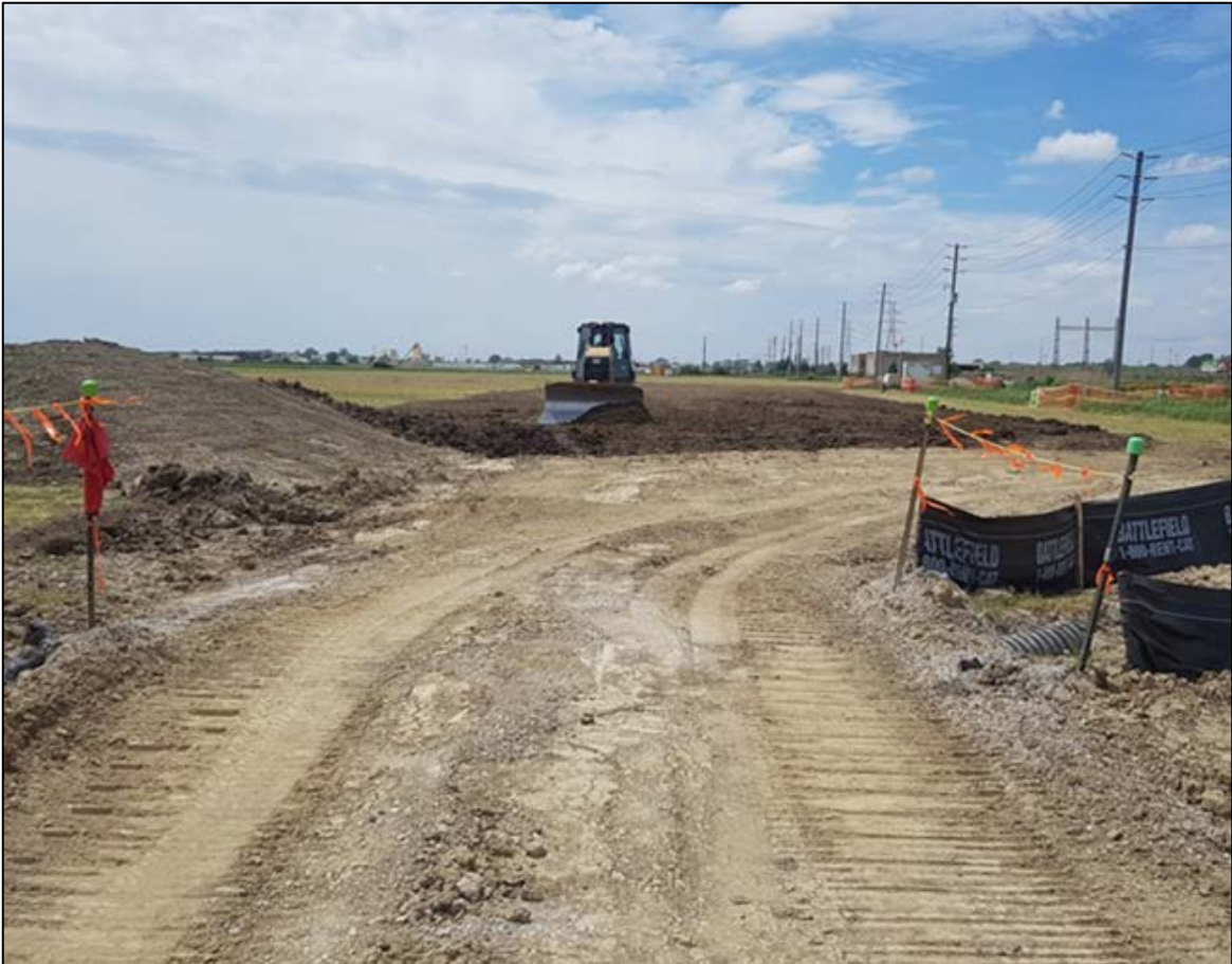
8. Spreading topsoil evenly across the work area on the agricultural field during clean up.
