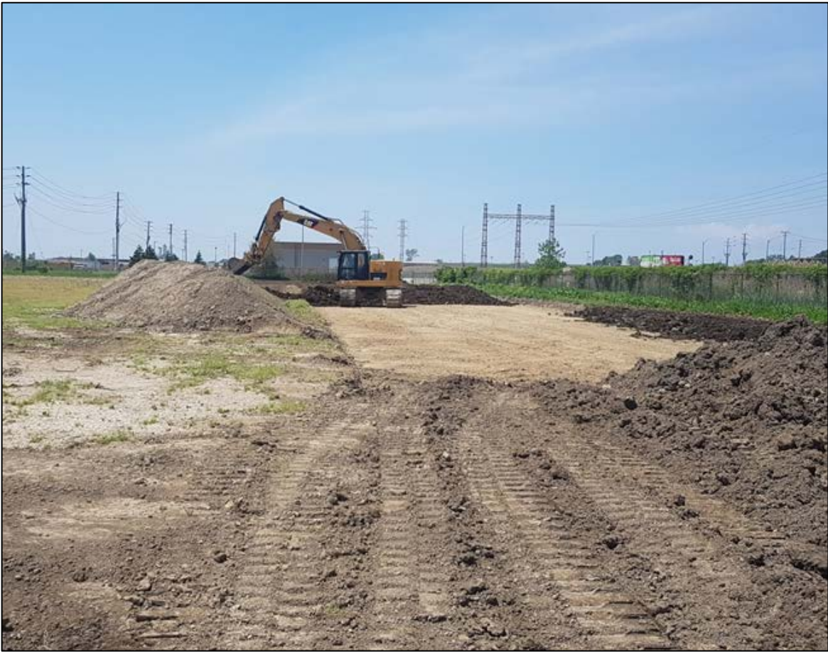
7. Pulling the stockpiled topsoil back on to the work area during clean up to restore the agricultural land to its previous state.
