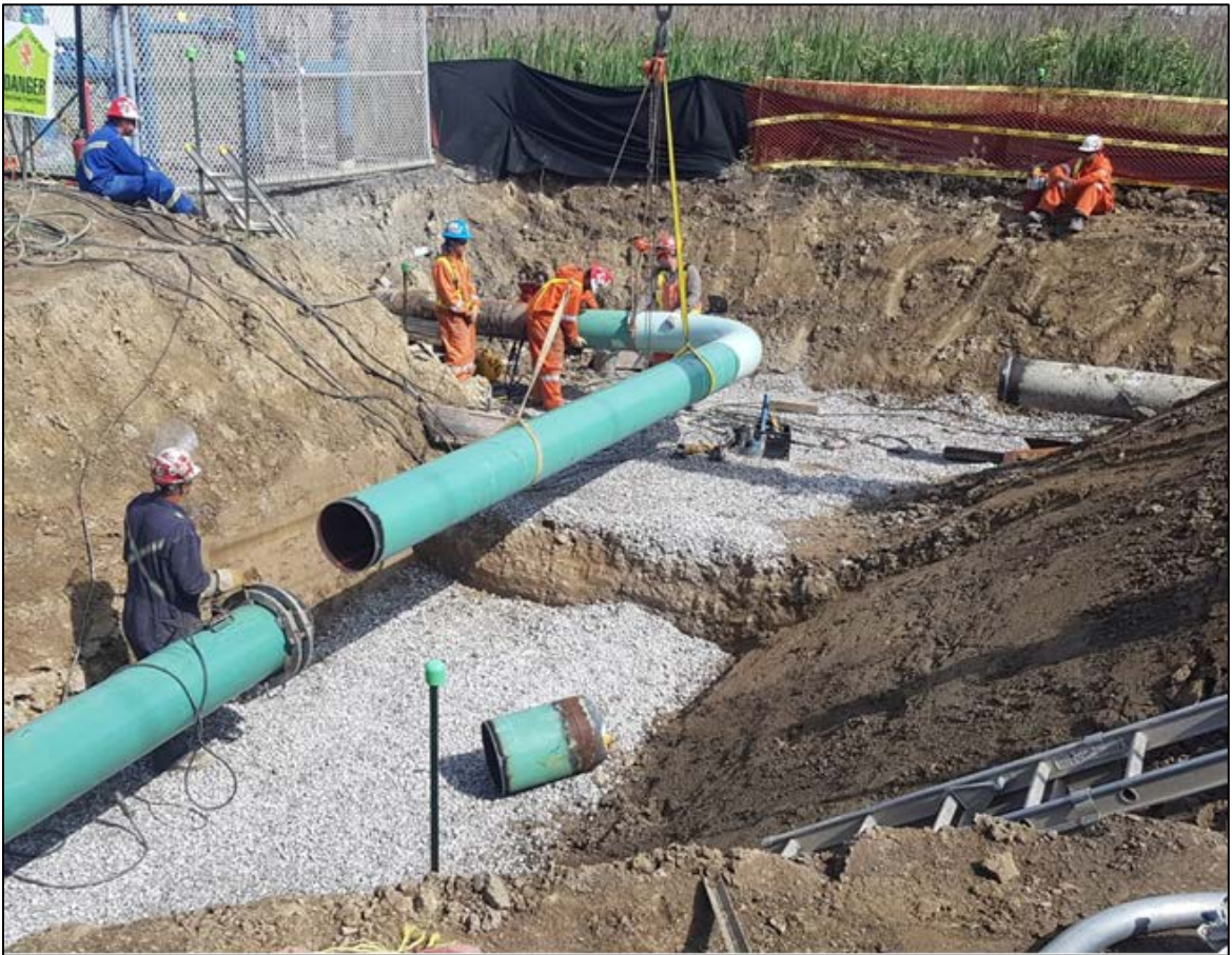
6. Tying-in the new 16" pipe to the existing pipe (left) and abandoning the old 16" pipe (right).
