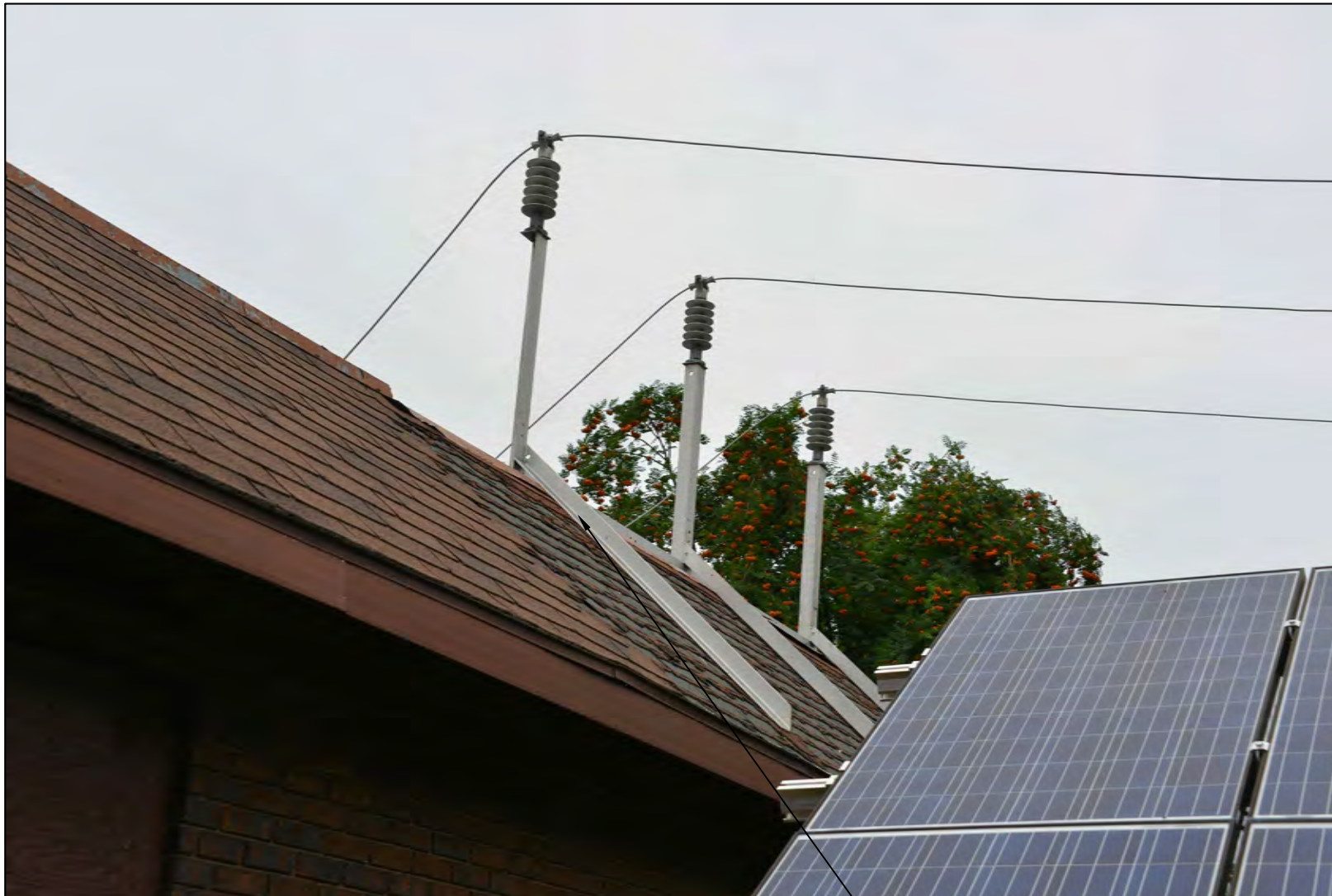
HOME-MADE 44KV SUPPORTS ON ROOF. ENGINEERING REVIEW REQUIRED.
