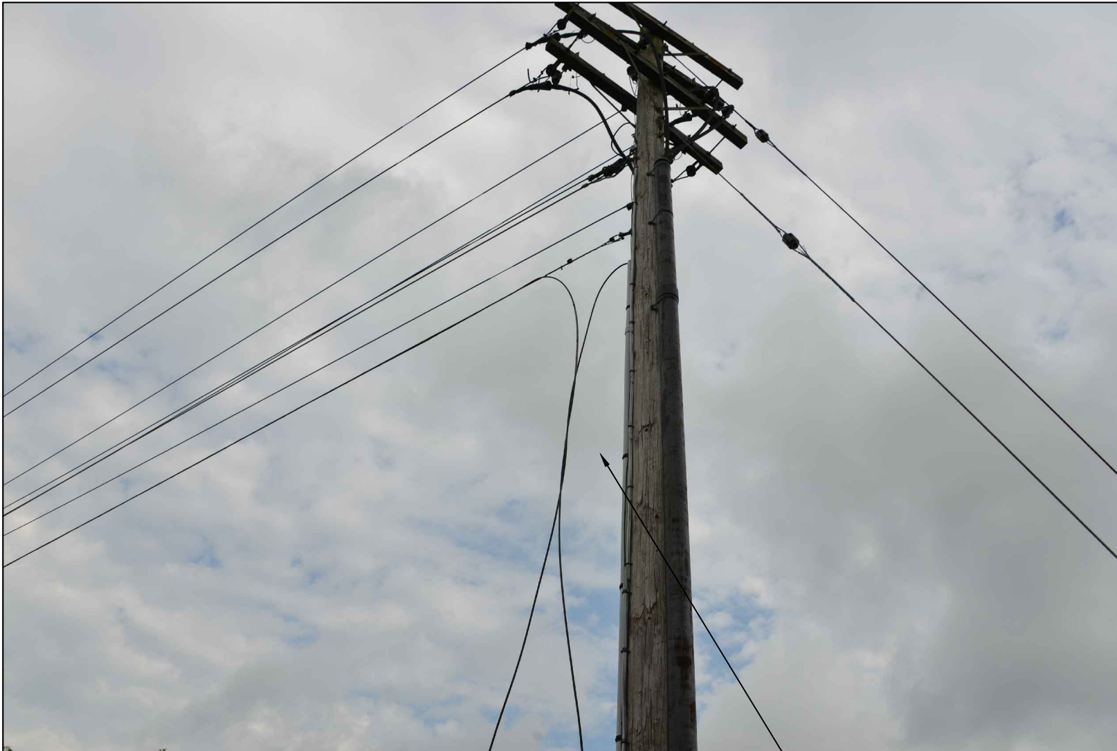
TELECOM CABLE HANGING DOWN
