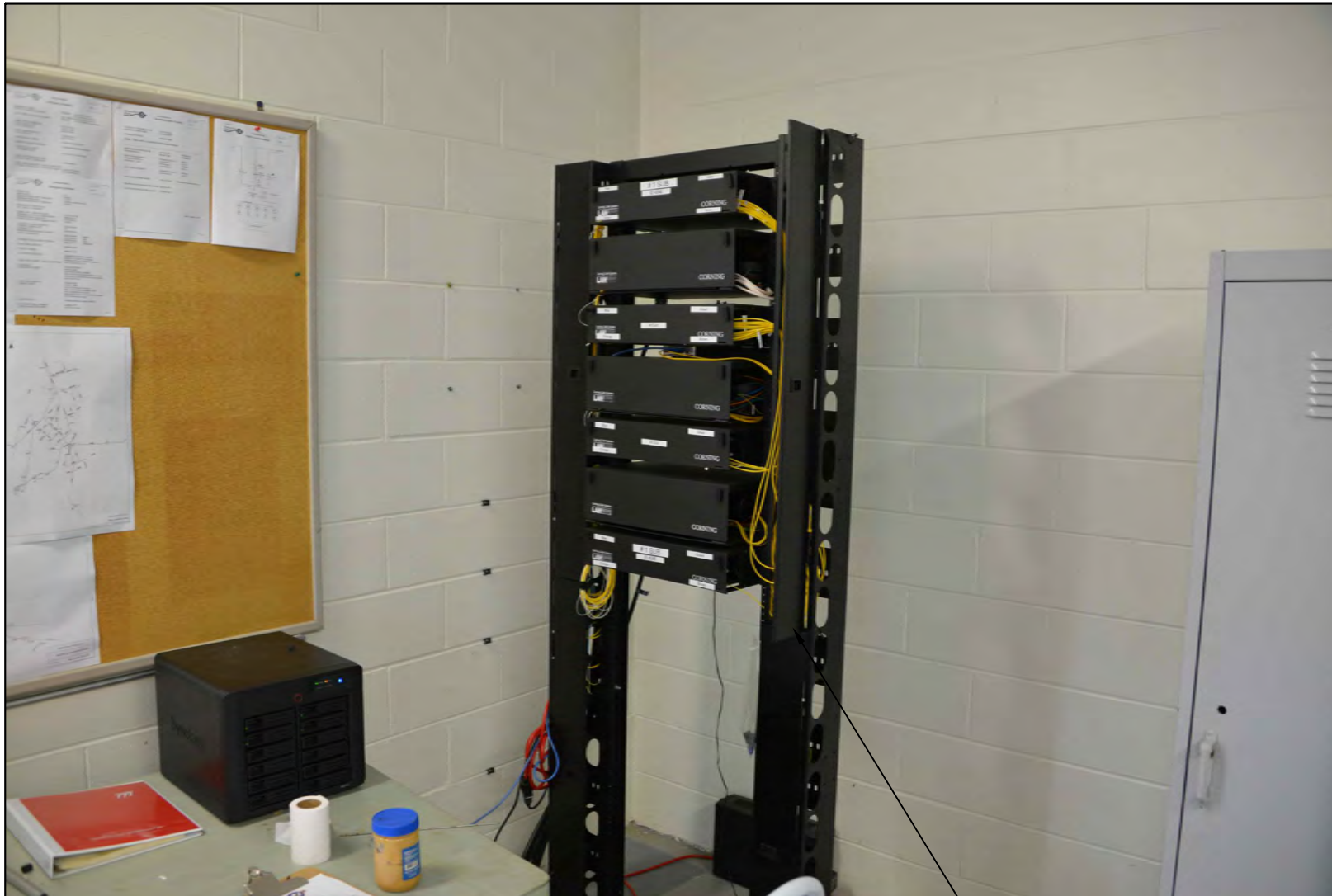
TELECOM EQUIPMENT IN SUBSTATION.
