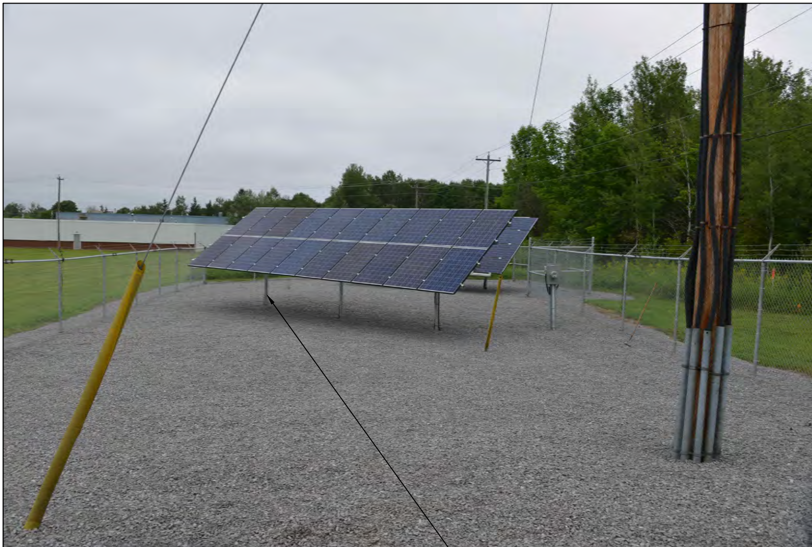
POSSIBLE GROUNDING AND BONDING ISSUES ON SOLAR INSTALLATION
