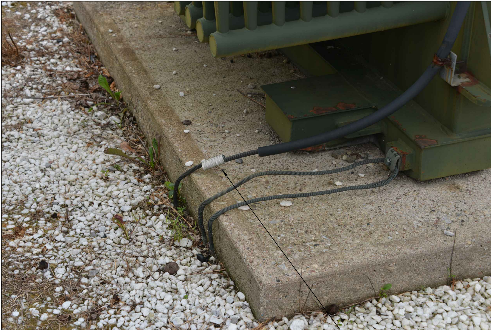
IMPROPER CONNECTION ON XO GROUND
