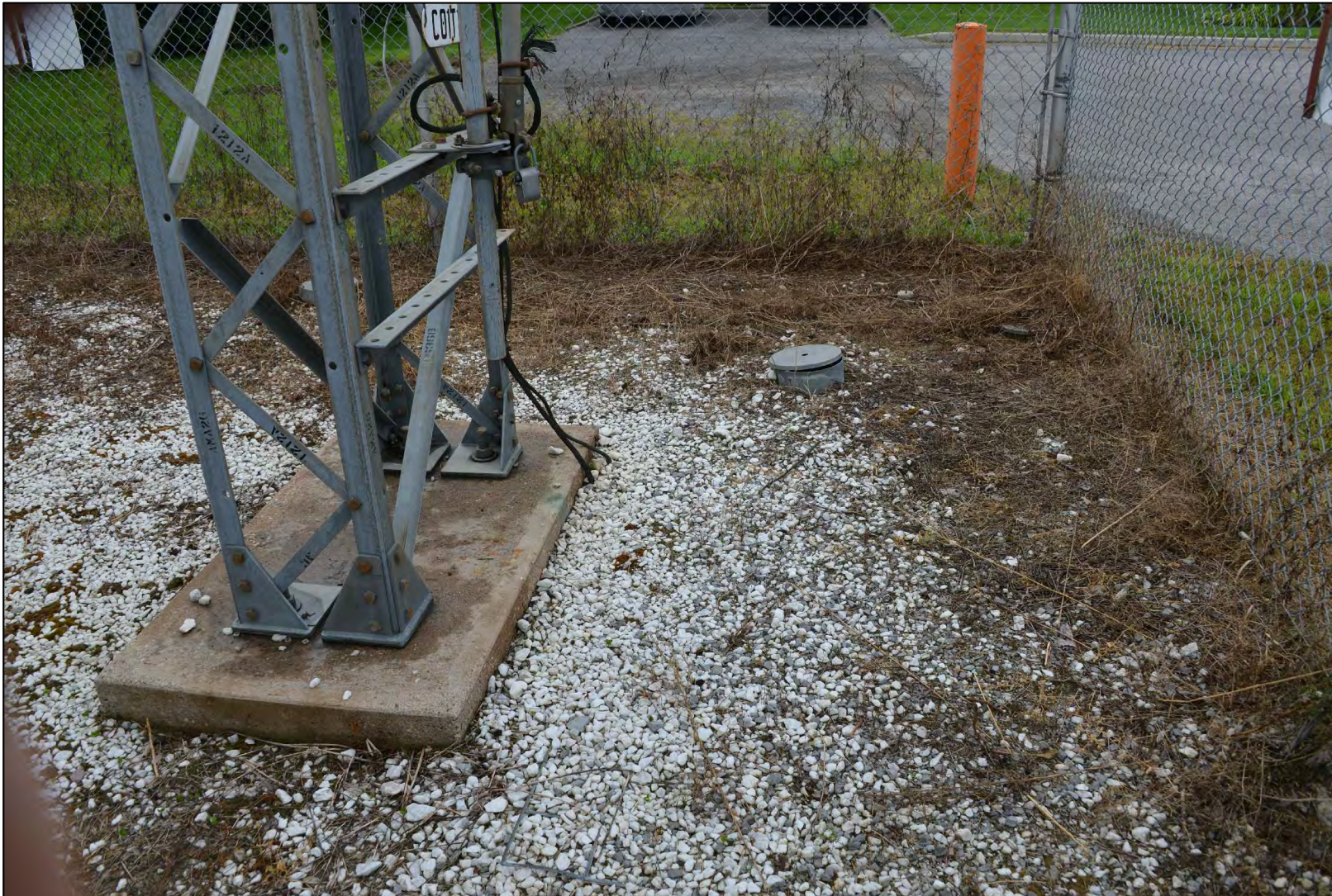
POOR YARD CONDITION
