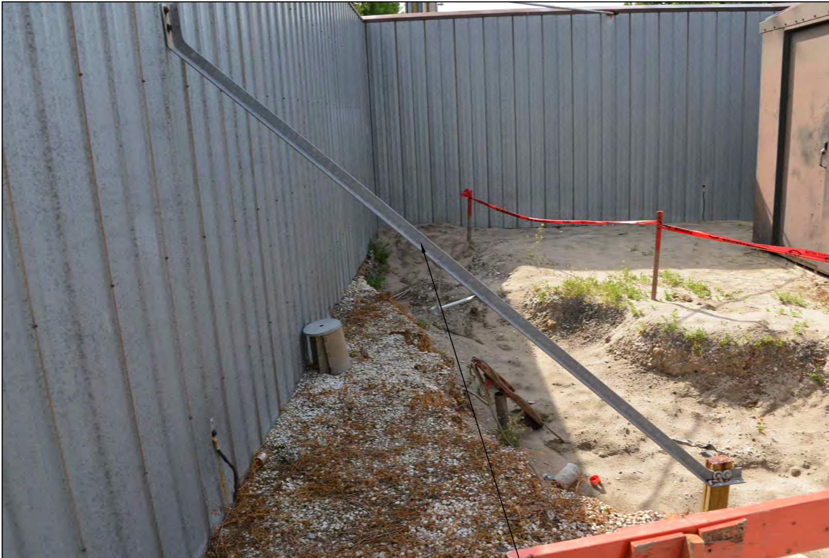
BRACING FOR UNSTABLE WALLS. NO GROUNDING, NO ENG. REVIEW
