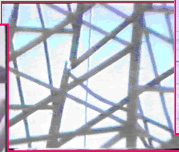
TOWER MAIN LEG BROKEN DURING GALLOPING
