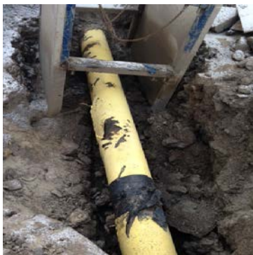
Figure 5.2-25: Gouges and dents due to latent damages
