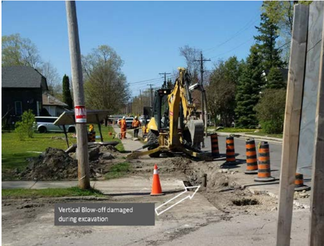
Figure 5.2-4: A Shallow Vertical Blow-off Assembly Damaged during Excavation
