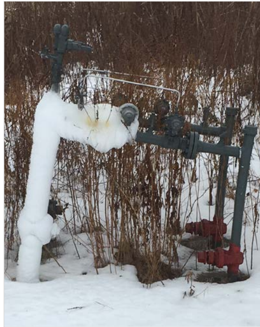
Figure 5.3-10: The Joule-Thomson Effect on a District Station
