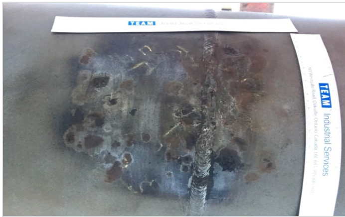
Figure 5.2-21: NPS 20 KOL Pipeline Displaying 70% Wall Loss Identified by ILI in 2016
