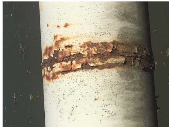
Figure 5.2-23: NPS 20 Pipe Crossing Exhibiting Corrosion
