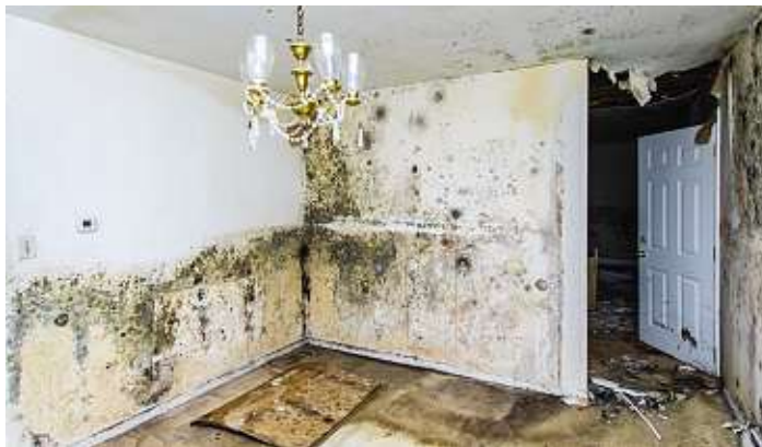
Mould can not only create extensive damage to your home, it can cause serious health problems. GETTY IMAGES
