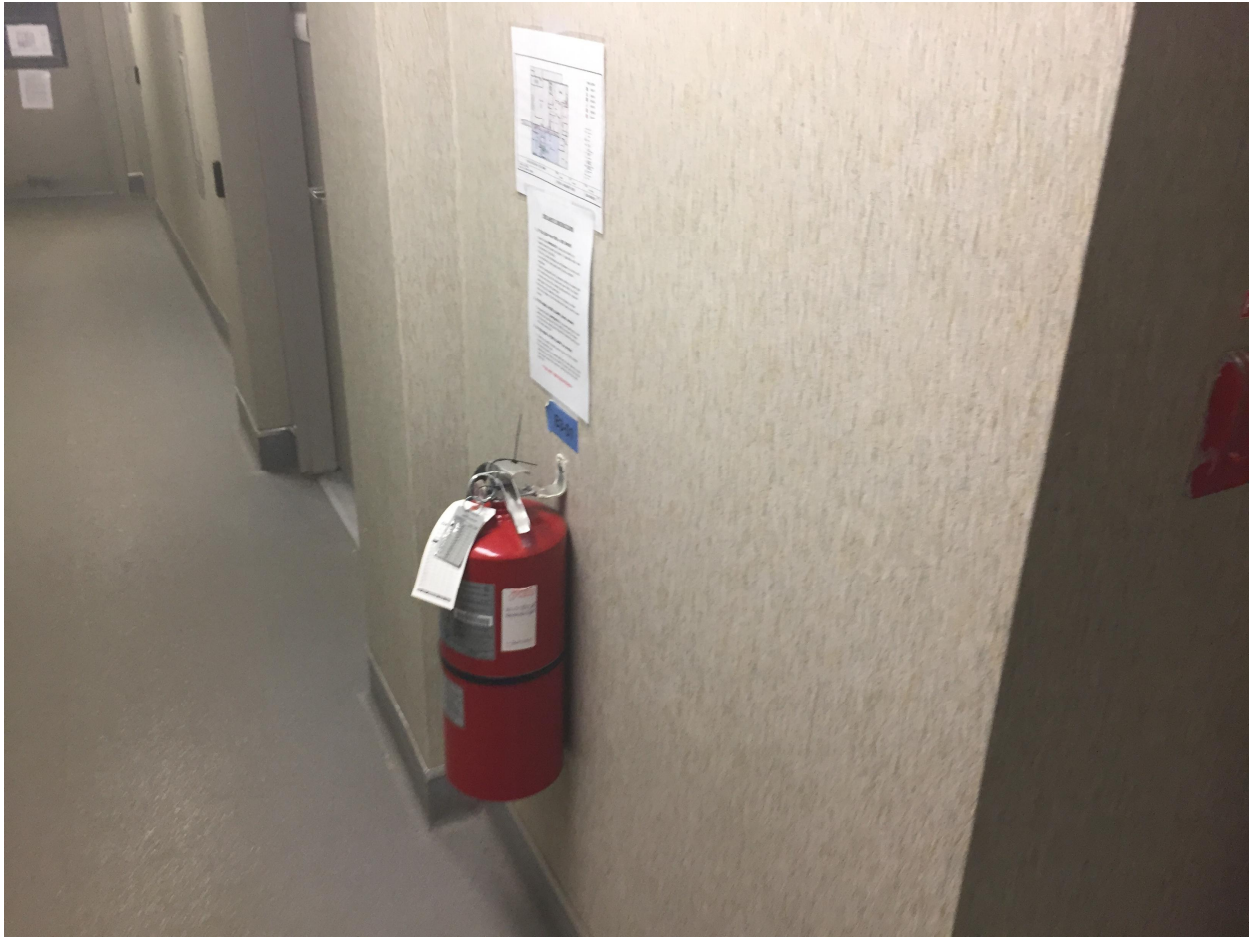
Suite 'B' Basement Photo 8 – Photo taken in the corridor of a fire extinguisher. There are extinguishers throughout the facility. Each is checked and certified annually as can be noted by the tag.
