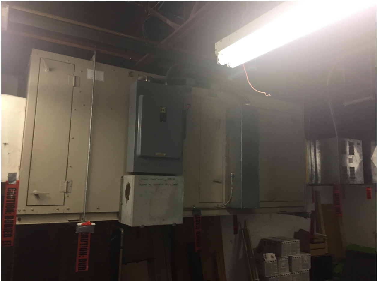
Suite 'B' Basement Photo 10 – HRU unit installed in 1994. This unit is now going on its 25 years. Presently the system is in good working order. However there can not be a determination on its life expectancy.
