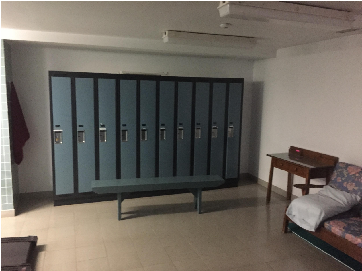
Suite 'B' Basement Photo 3 – Entrance to Woman's washroom / change room / shower. Comfort area and lockers.
