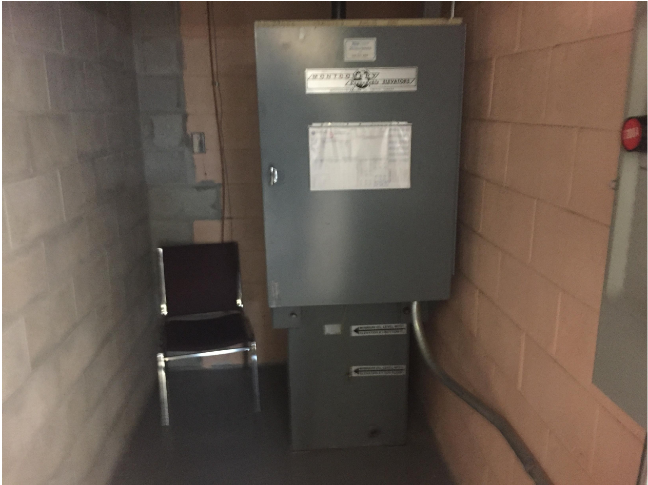
Suite 'B' Basement Photo 15 – Suite 'B' is also served by a freight elevator. This elevator on rare occasions is used for individuals with mobility issues. Photo of Elevator mechanical equipment and main disconnect.
