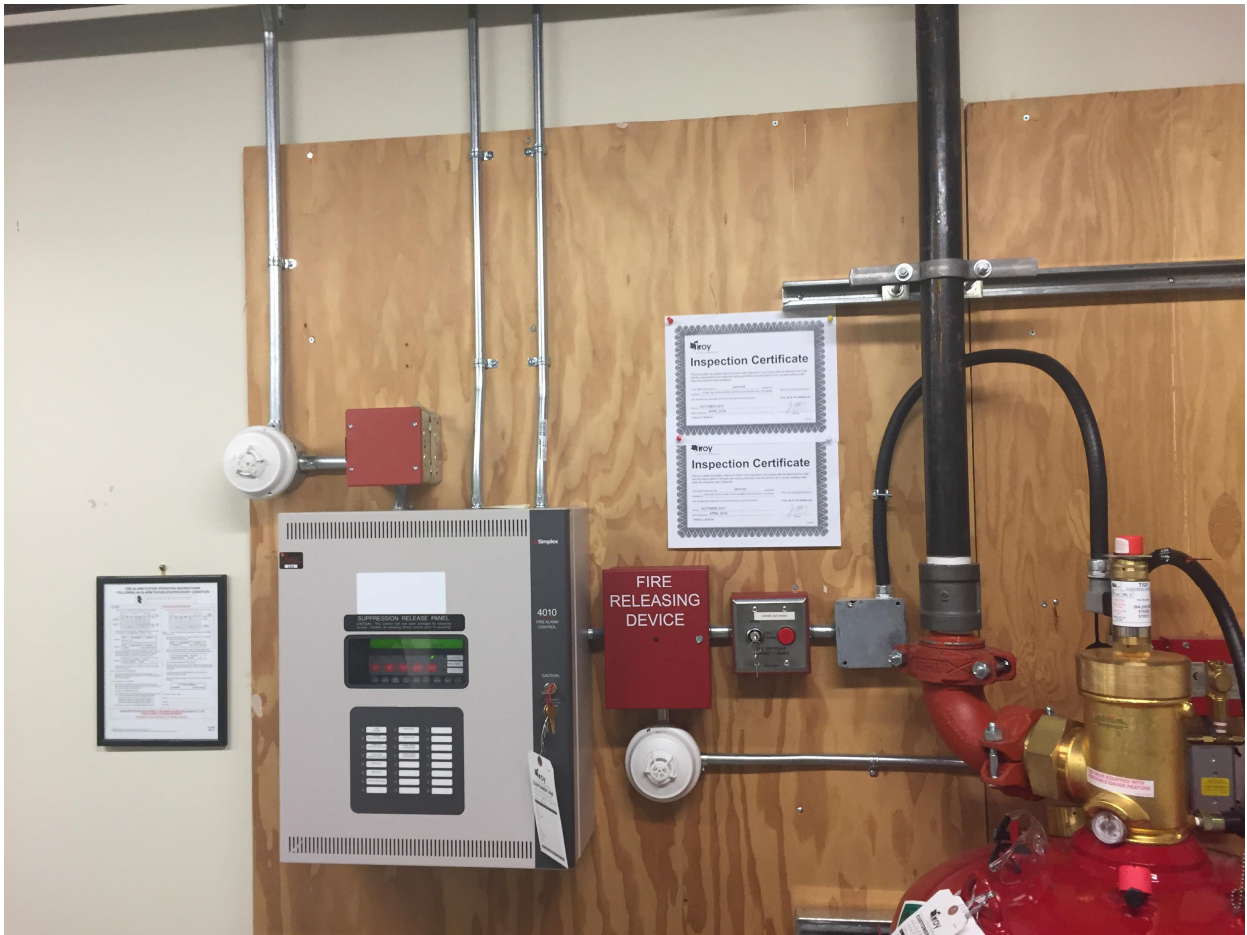
Suite 'B' Basement Photo 16 – Suite 'B' does not contain a sprinkler system, however it does contain a "Dry Chemical" suppression system located within the basement in their general server room.
