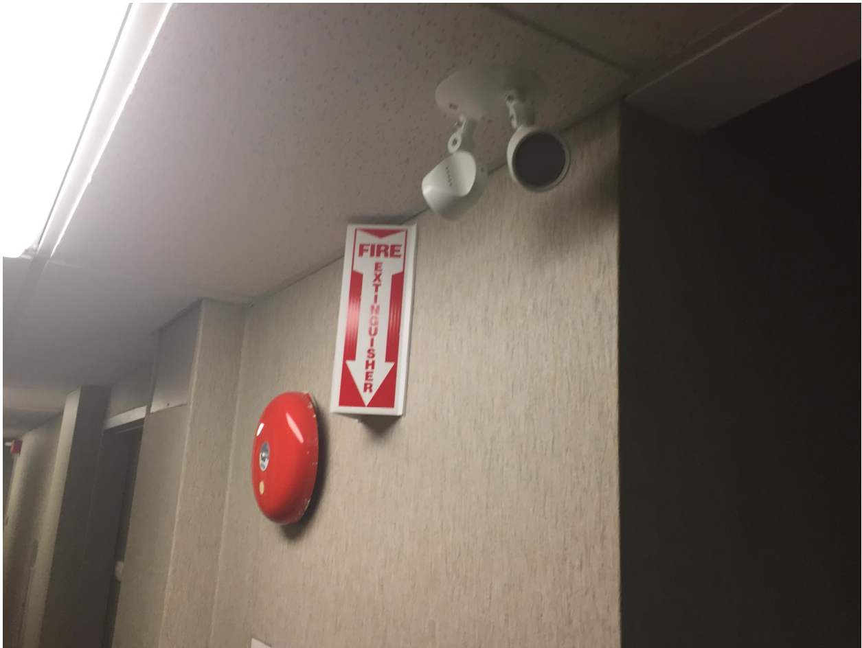
Suite 'B' Basement Photo 9 – Photo taken in the corridor of an alarm bell. There are alarm bells throughout the facility. Each is checked and certified annually.
