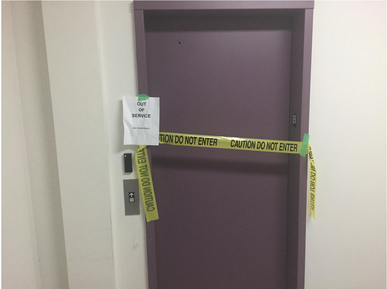
Suite 'A' Photo 9 – Passenger Elevator. Due to mechanical issues the elevator has been temporarily taken out of service.
