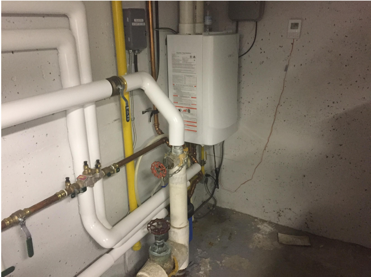
Suite 'B' Basement Photo 11 – Primary source of domestic hot water is a “On Demand” gas fired water heater manufacture by ‘NAVIEN’. Date of installation is unknown.
