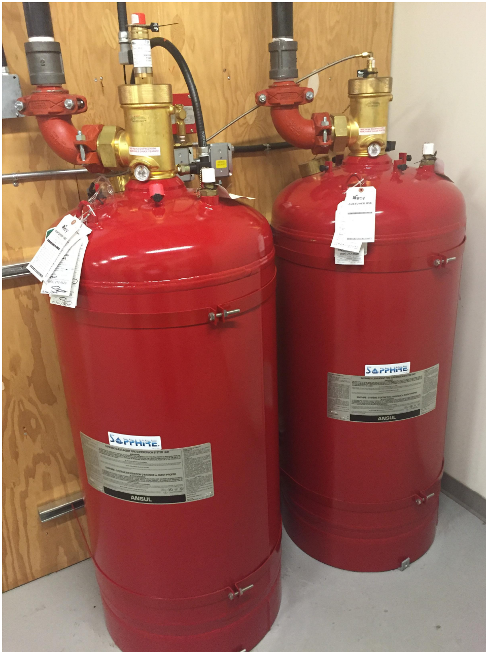
Suite 'B' Basement Photo 17 – “Dry Chemical” suppression system located within the basement in their general server room. See photo 16.
