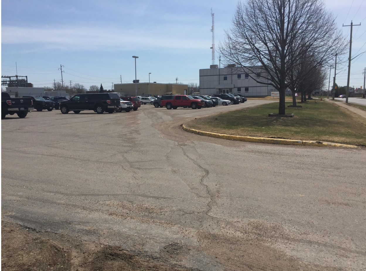
General Site - Photo 2 – Second Entrance of Main parking area – Looking South. There is obvious settlement of the soils of the parking area around the main storm drain. There is ‘alligating’ and patches in the parking main area.
