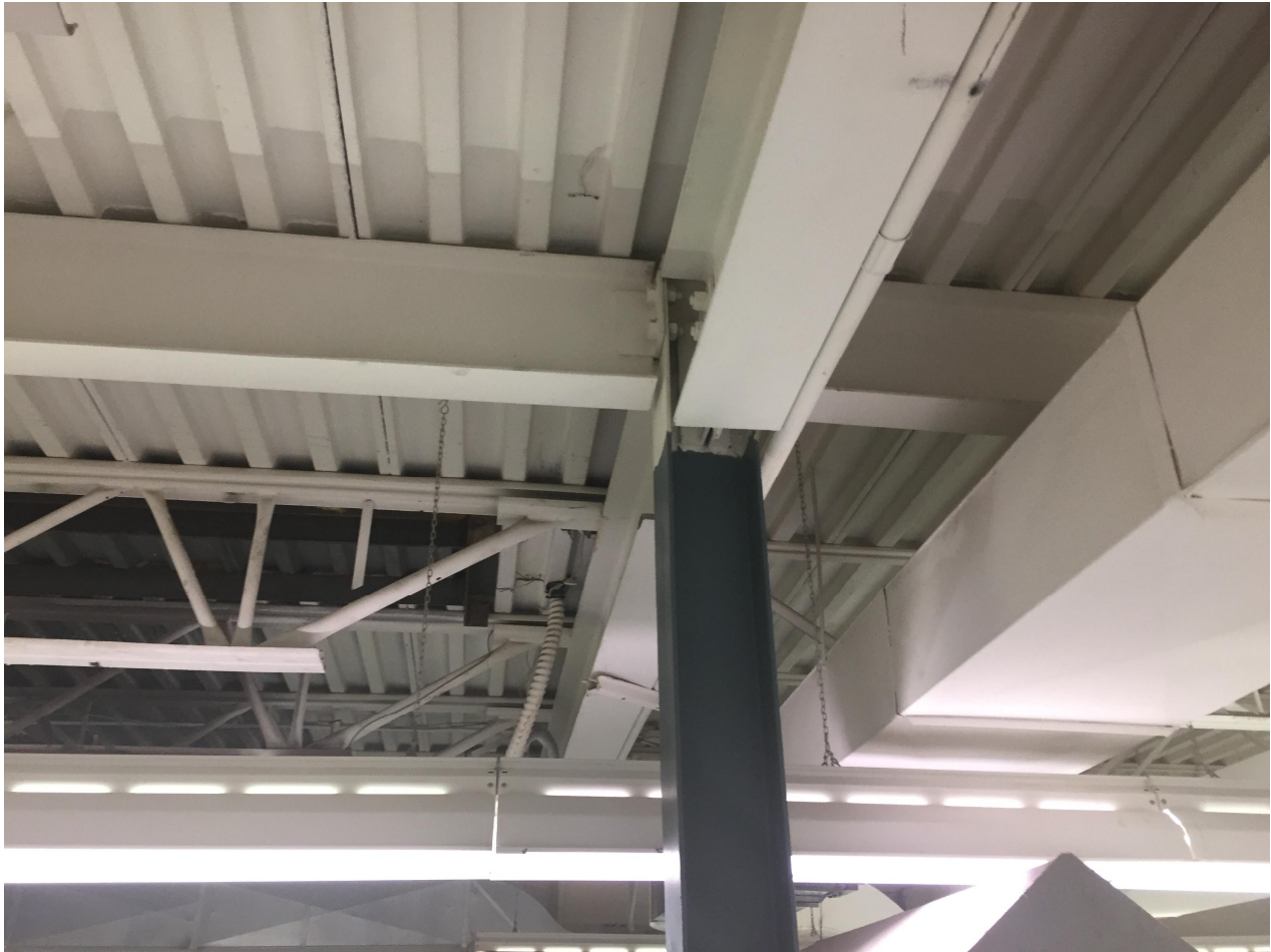
Suite 'B' Basement Photo 7 – General floor construction (first floor / basement ceiling) consisting of OWSJ and metal deck and a series of steel columns.
