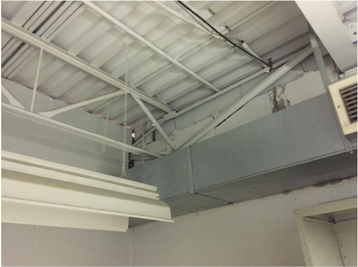
Suite 'B' Basement Photo 4 – General floor construction (first floor / basement ceiling) consisting of OWSJ and metal deck. Concrete block partition walls can also be observed.
