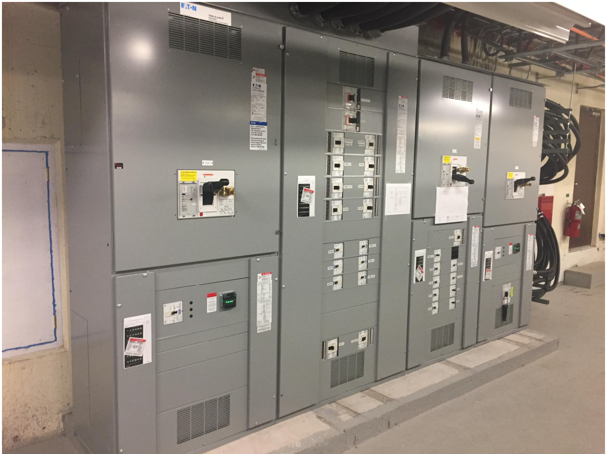
Suite 'B' Basement Photo 19 – Main electrical, switch gear and disconnects located in the server / electrical room. The power enters underground from a pad mounted transformer located on the south east of the property. 1600amp service is provided. Remainder of facility and suites are served and distributed from this main service.
