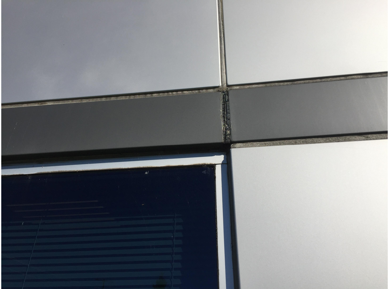
Suite 'A' – Suite 'B' Typical Exterior – Photo No.3 - Exterior view of the exterior aluminum panel system and caulking failure. A coloration seemed to exist between the accent band (brown color panel) and the location of leaks. It may be hypothesized that the color of the caulking or its chemical makeup was not as resilient as the lighter shade of caulking.
