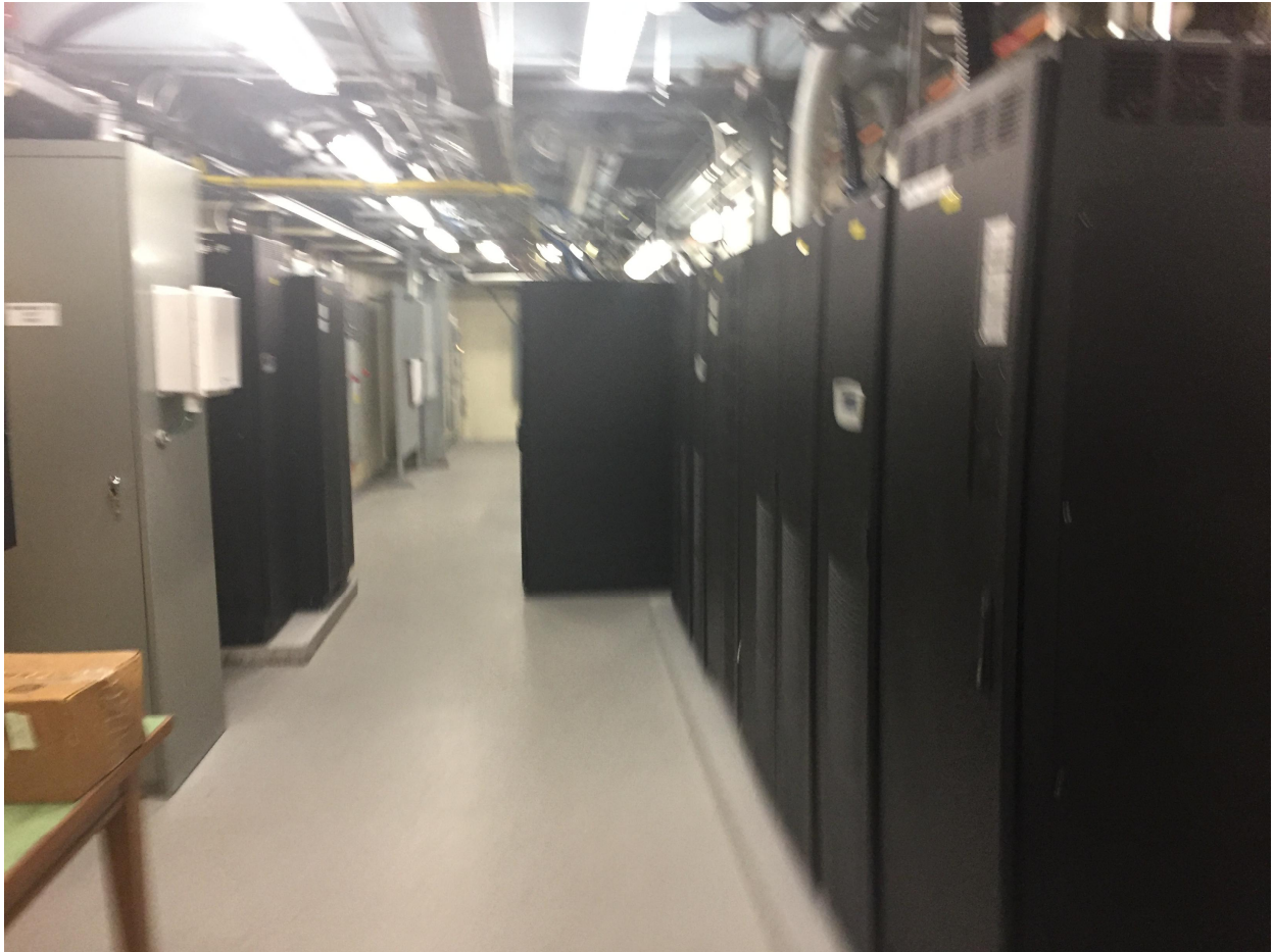
Suite 'B' Basement Photo 18 – General server and electrical room, located within the basement.
