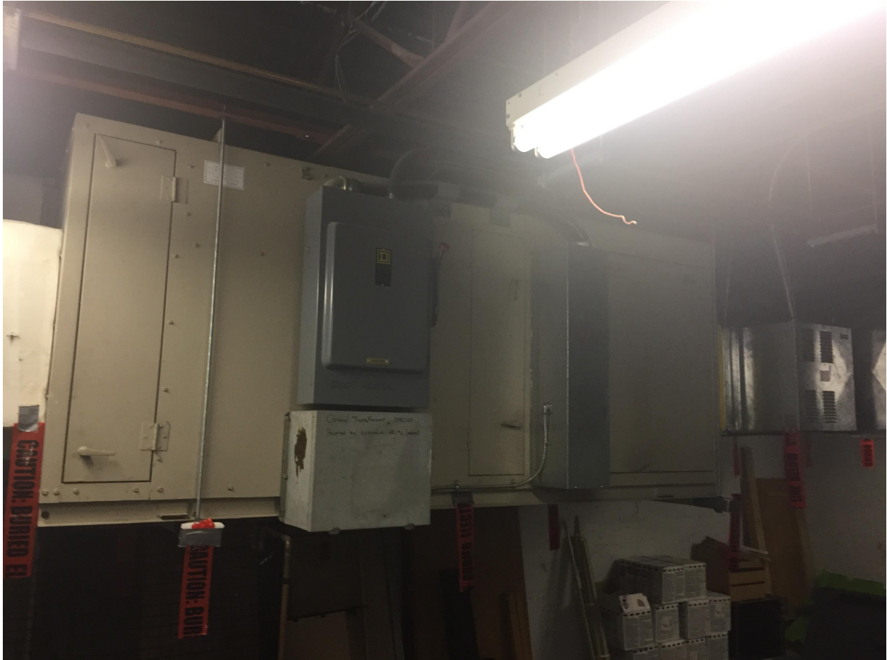
Suite 'A' & Suite 'B' Basement Photo 5 – HRU unit installed in 1994. This unit is now going on its 25 years. Presently the system is in good working order. However, there cannot be a determination on its life expectancy.
