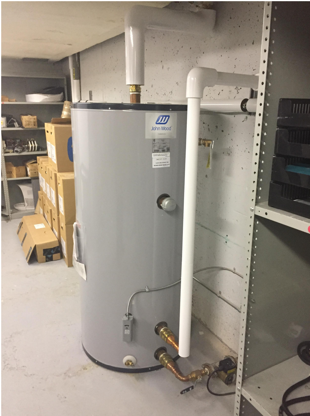
Suite 'B' Basement Photo 12 – Secondary source of domestic hot water is a traditional electric hot water tank. Date of installation is unknown.
