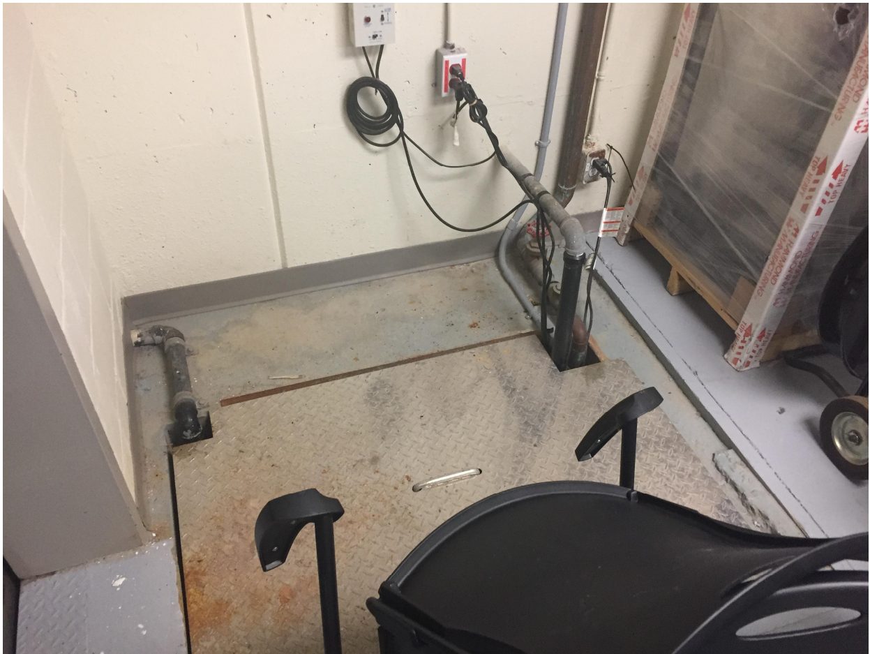
Suite 'B' Basement Photo 13 – Main sump hole complete with pump. There are two sump locations in the basement of Suite 'B'. Both are monitored and are connected into the storm water system.
