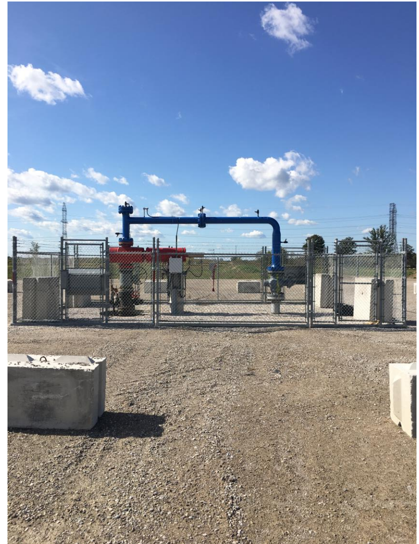
Figure 11: TD28H looking West
