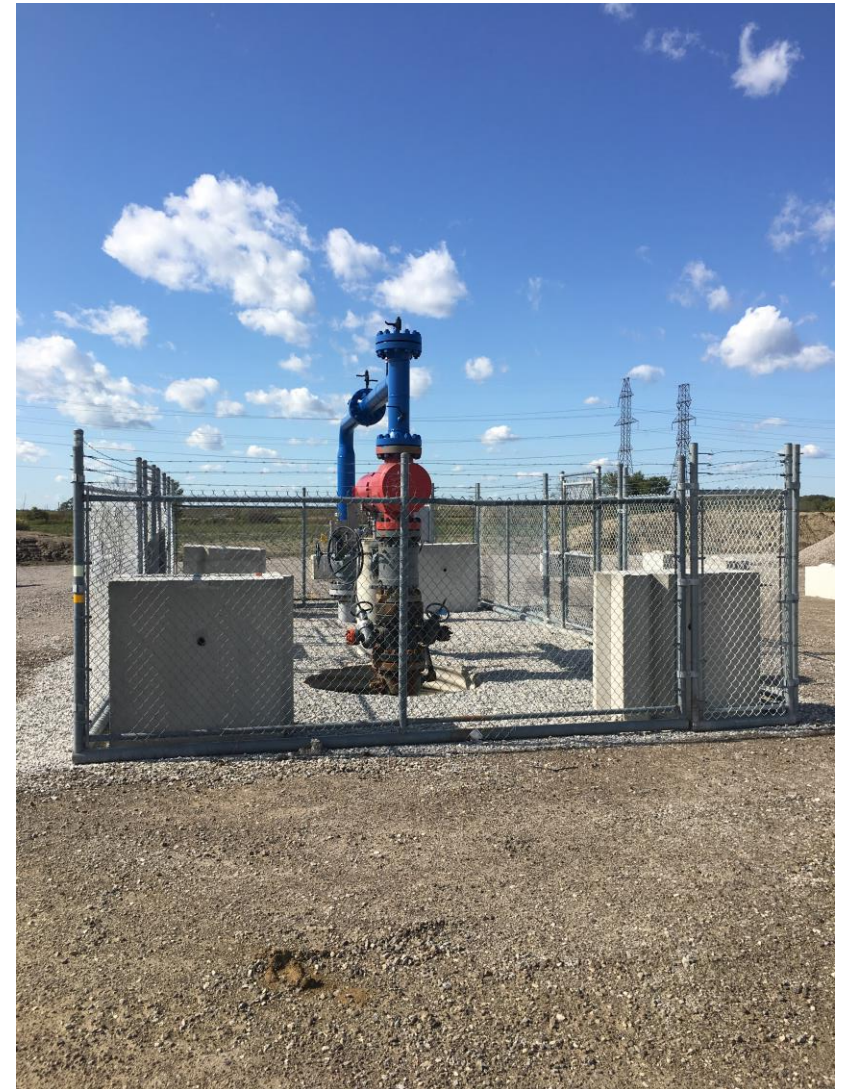
Figure 15:TD29H looking West
