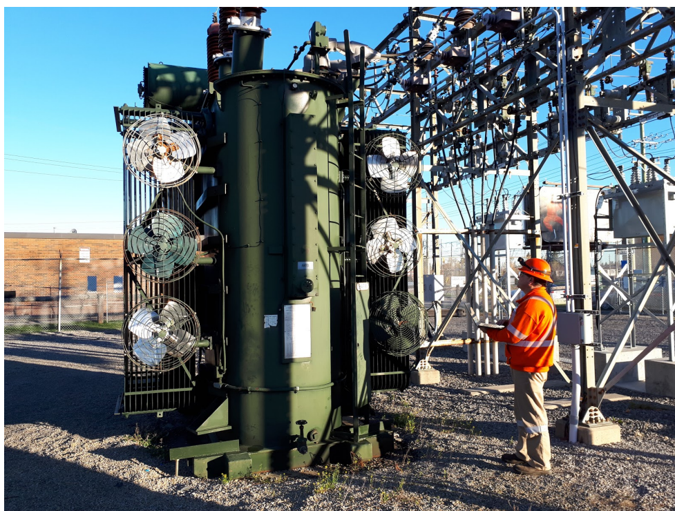
14 15 Figure 6.51 – Visual Inspection of a Station Transformer
