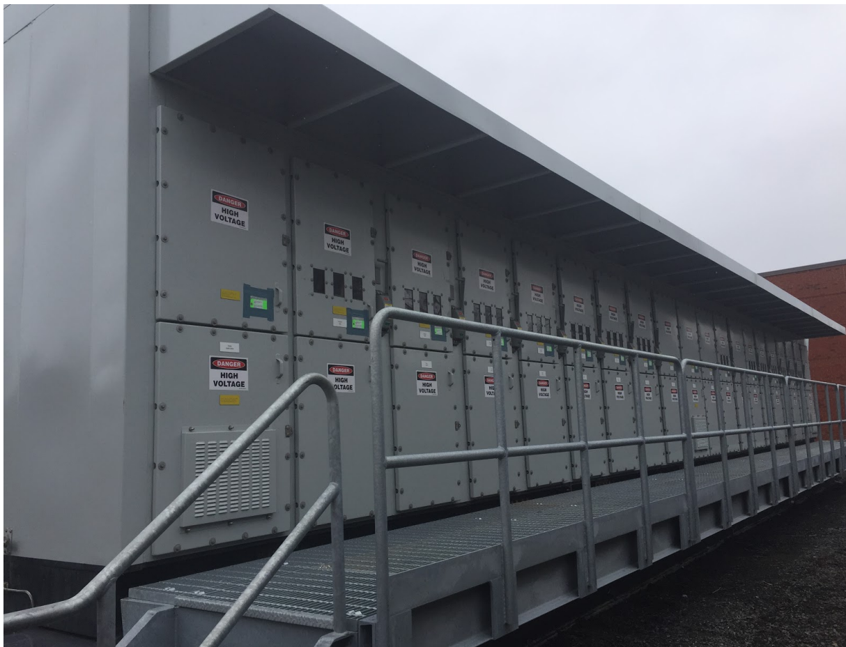
Figure 6.8 – Station Switchgear at Woodroffe TS
