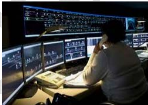
The image below shows a typical view of a control room set-up.
