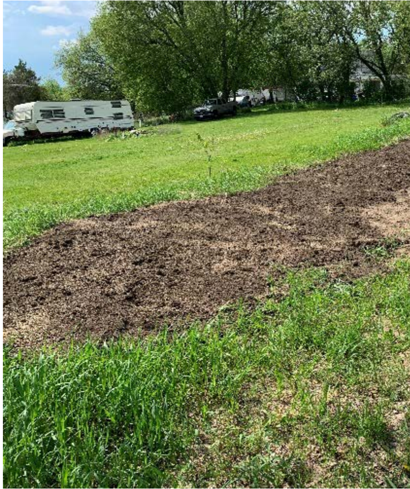
Photo 3: Topsoil and seed placed on sandy embankment just south of Flos Road 8.
